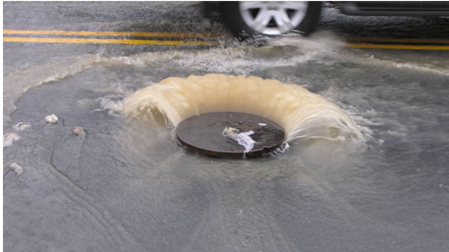
Figure 1.1 CSO on Platt Avenue in West Haven, Connecticut, April 23, 2006 (Zurcher, 2006)
