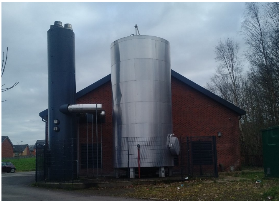
Figure 6.2: WWHC hot water tank and flue chimney in foreground, and boiler house in background
