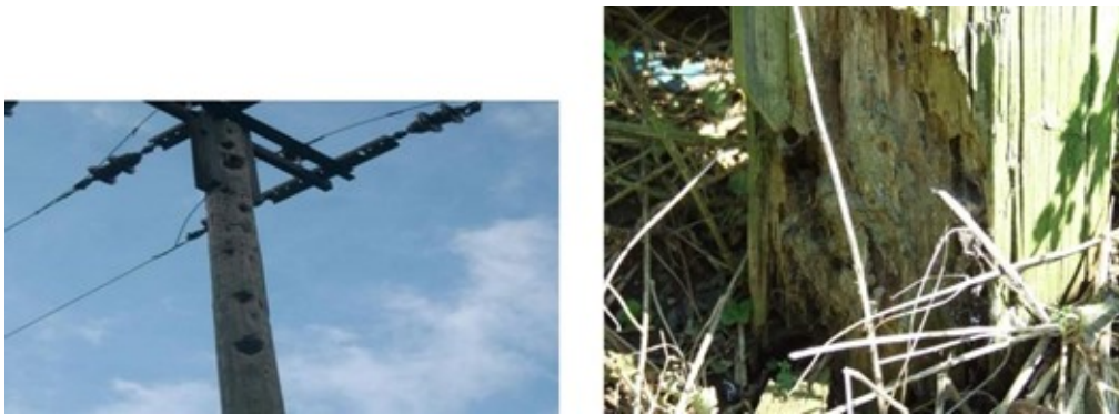
Figure 2.4: (UK Power Networks) Woodpecker damage (left), Pole rot (right).
