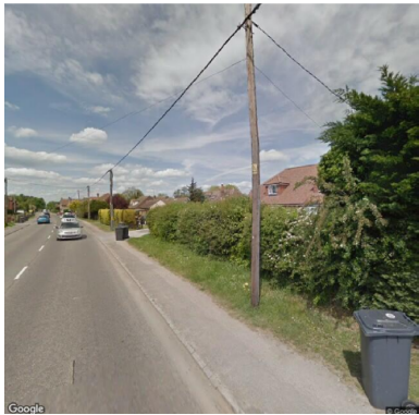
(a) Wooden Utility Pole.
