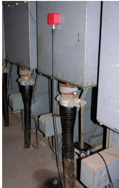
Figure 5: Photo of TEV Sensor Attachment to Cable Box & HFCT connection to Cable Earth Bar
