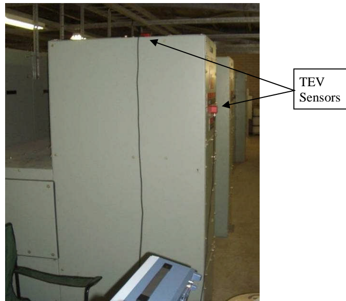
Figure 11: Placement of 2xTEV Sensors on Switchgear Panel for TOF Measurements
