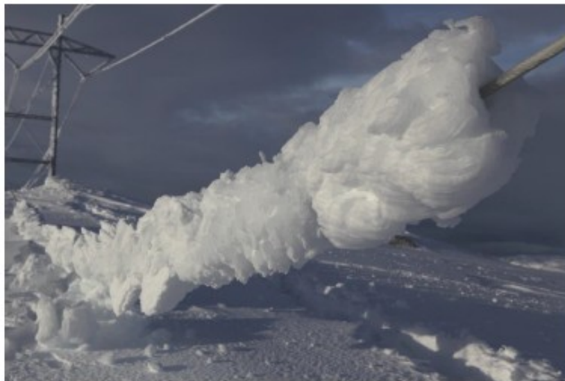
Figure 2.6: Accumulated ice on a broken ground wire, January 2014 [7]
