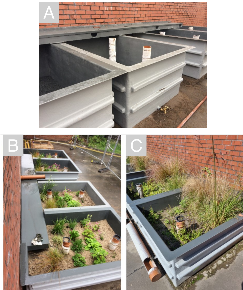
Figure 5.1: Rain gardens on Washington Street, Glasgow prior to the addition of soil and plants (A), shortly after installation in 2019 (B), and in 2021 (C). Photos B and C by Civic Engineers.
