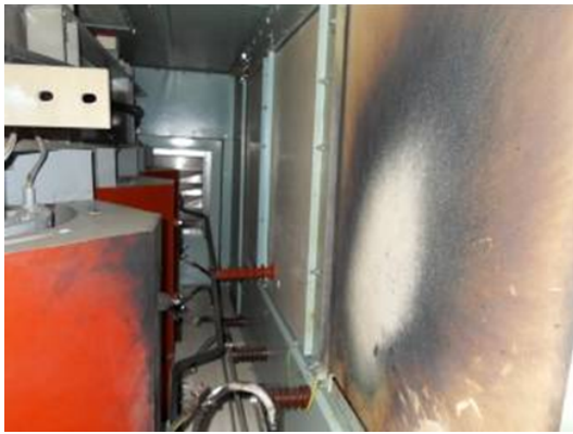
(a) Evidence of vaporised conductor due to an arcing fault on a marine vessel transformer [Daf09]
