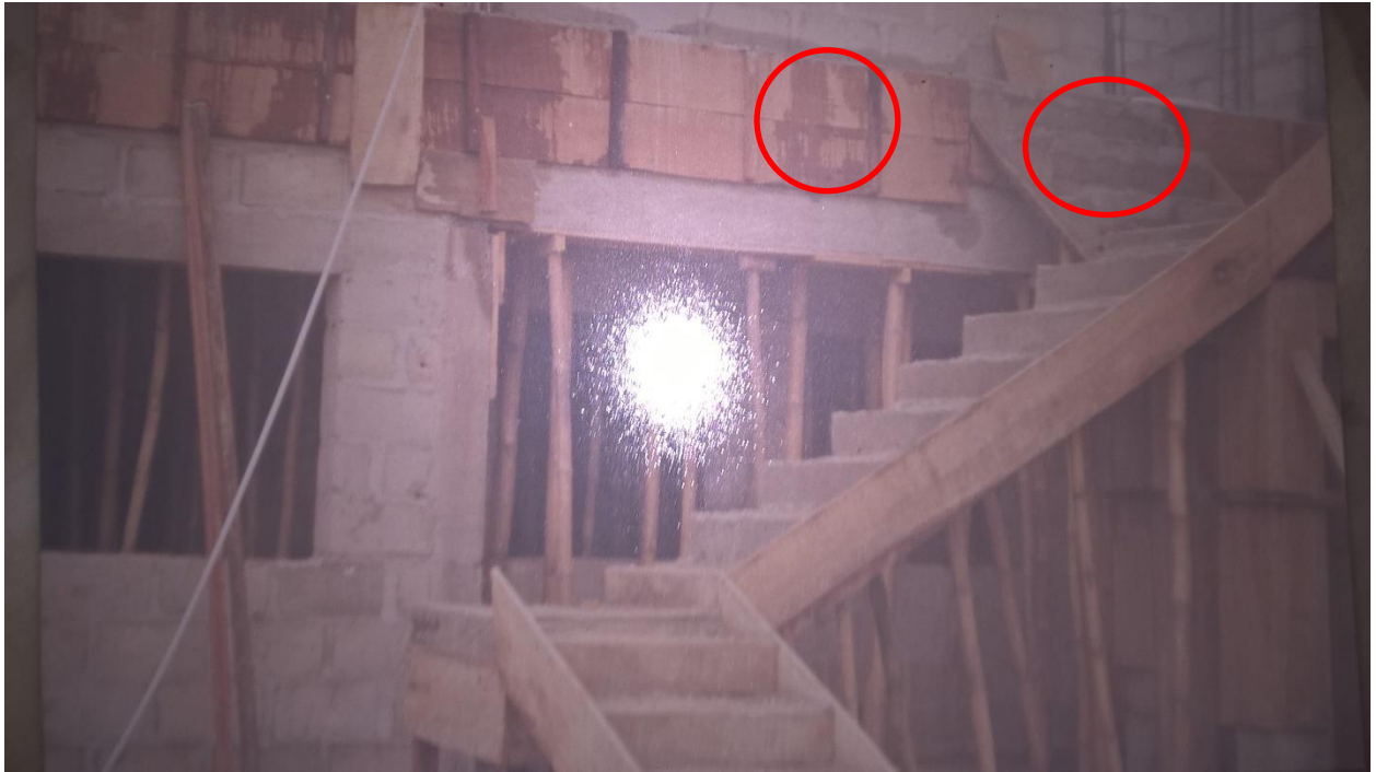
2 nd floor manual concrete placement and unprofessional staircase construction
