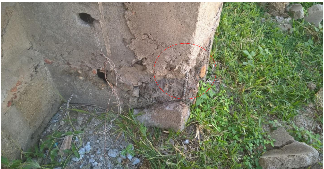
Figure 4.11: Unprofessional practice of reinforcement rod exposed
