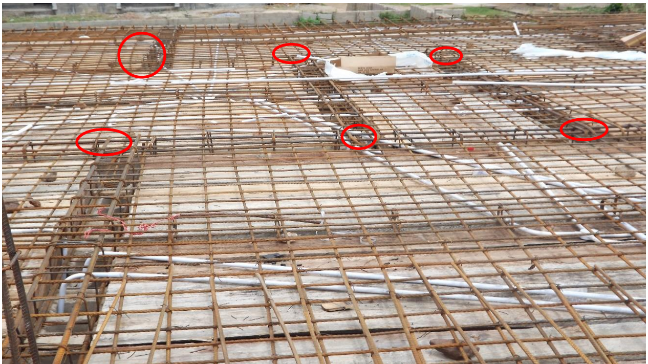
Figure 4.9: A display of non-compliance with structural design in column placement
