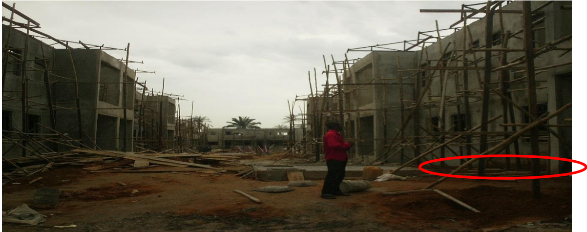
Example of MRRB: 2 Bedroom Semi-Detached Residential Building with Low floor level therefore possibility of dampness to weakling the foundation
