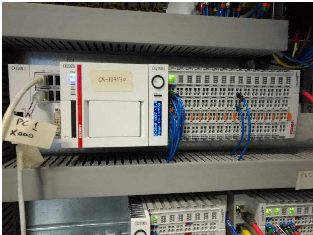
Figure 7-5. Beckhoff Industrial PC and IO's
