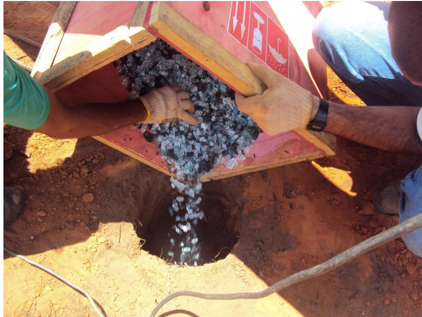
Figure 8.6: Manually excavated 2.5m deep, 25cm diameter borehole. The first 2m from bottom were filled with glass shards and the remaining 0.5m with soil. The glass shard pile was exactly below the hydraulic jack.
