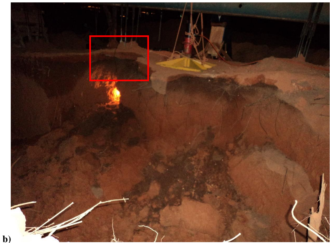
Figure 8.16: Photos of FT3 No4 failure event during Experiment L1 before (a) and after (b) with the soil block that fell inside the excavation indicated with a red box.
