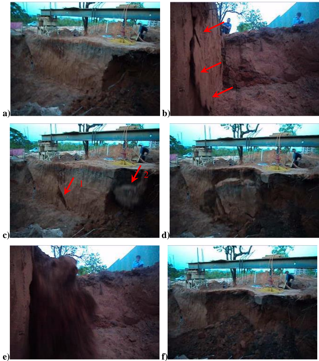
Figure 8.15: The FT2 No2 failure event (FT2: soil block topple and fall), L1 Experiment. (a) VF1 after Failure 1, (b) Crack just before FT2 No2 took place, (c) Soil blocks 1&2 detached from VF1, that toppled and fell on the ground surface milliseconds before the main landslide failure event occurred. These events were considered part of the main Failure 2 event. (d, e) Main part of soil mass consisting FT2 No2, involving soil block topples and falls. FT2 No2 failure event along with FT2 No1 were the two largest failure event that occurred during Experiments L1 and L2.
