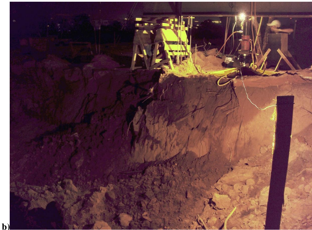
Figure 8.17: Photo before (a) and after (b) FT3 No.1 failure event of Experiment L2 (FT3: soil block fall). This was the biggest failure event occurring in this slope and the biggest failure event of FT3.
