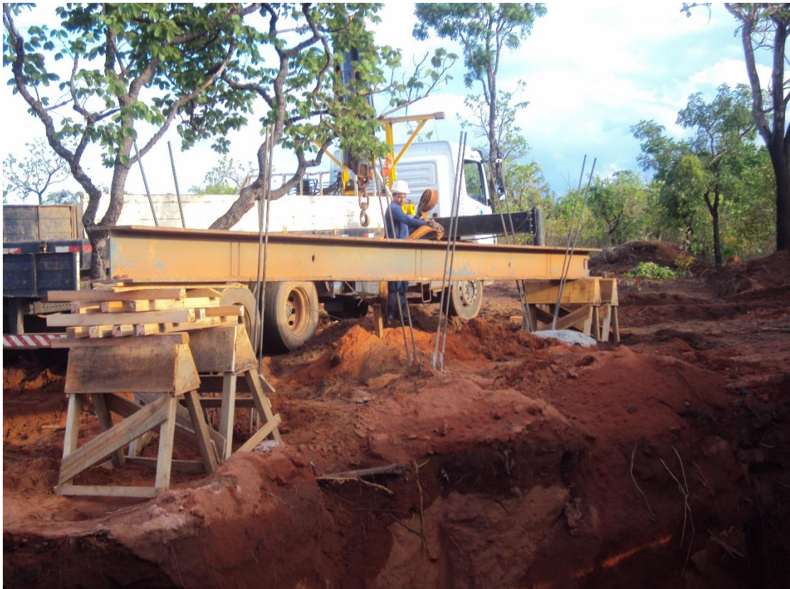
Figure 8.2: I shaped metallic beam placed on top of the three piles at a levelled position with two construction steel bars at either side of it. The weight of the beam was supported by four wooden stands, which restrained the beam from moving downwards. The wooden sticks on the left were used to keep the beam levelled.
