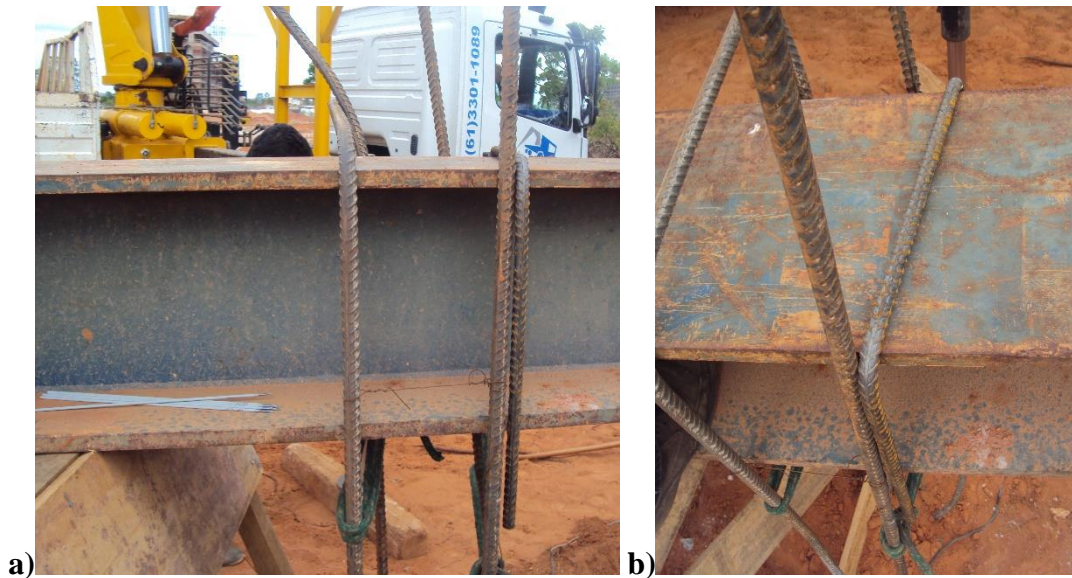
Figure 8.3: a) II shaped construction steel bars were used for welding two of the pile's construction steel bars on either side of the metallic beam. The II shaped bars were also welded on the beam. A total of 12 II shaped bars were used to weld the beam on the construction steel bars of all piles. After welding no vertical movement of the beam was possible.
