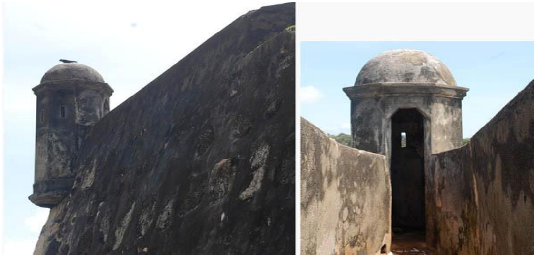
Figure 2.51 Turret at one of the bastions at the Galle fortress, 2009 (Source: Author)
