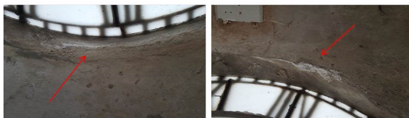
Figure 5.35: Efflorescence progressively fracturing the plaster render. Clock Tower window, west elevation.
