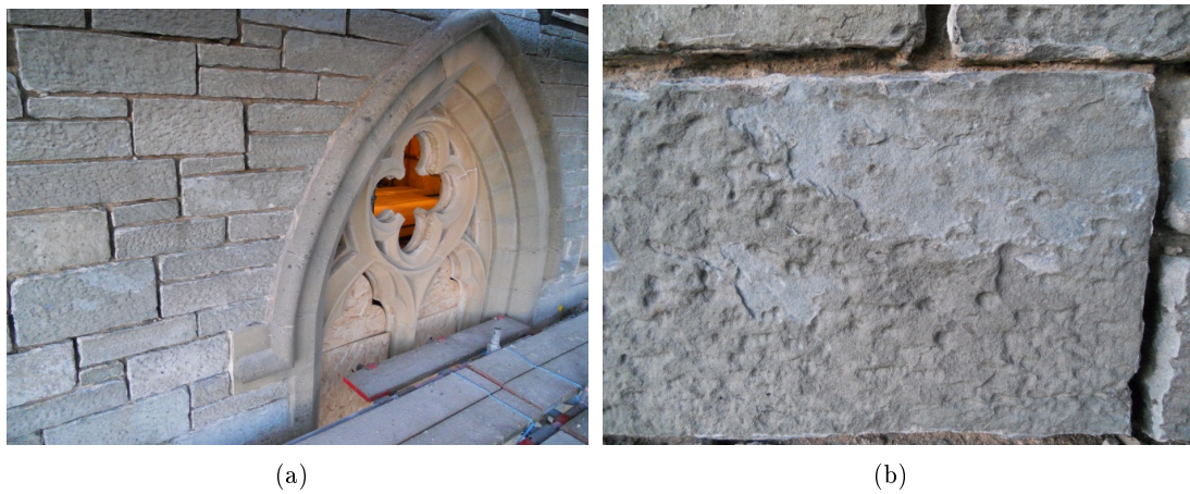
Figure 5.2: Image of the masonry beside the Lancet windows, Lerwick Town Hall (a) and detail of the deteriorated green sandstone (b).
