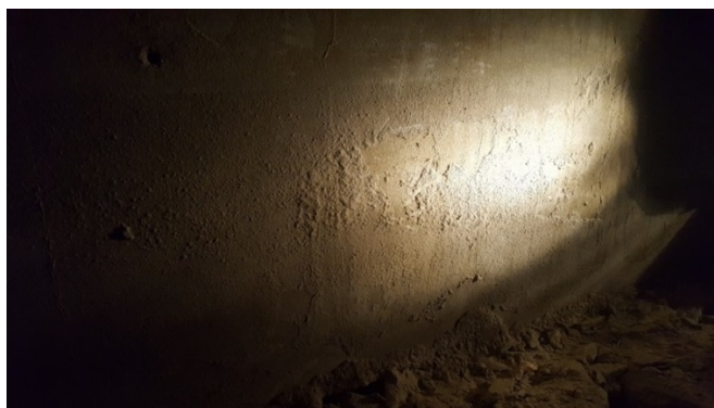
Figure 5.9: Light patina at the bottom of the right window (from inside) on the south side of first floor main hall.
