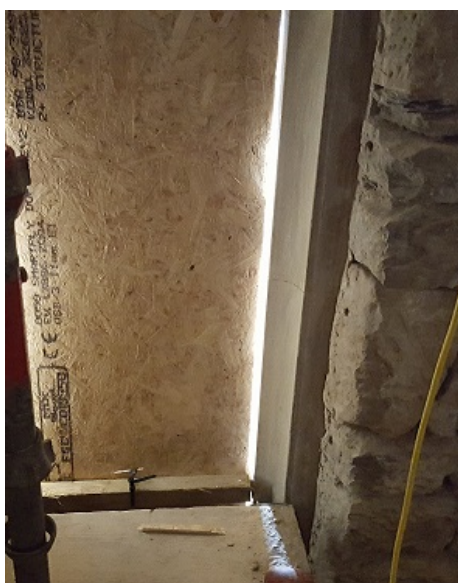
Figure 5.10: Area of sampling of SH10, on the middle of the right side of the right window (from inside) on the south side of main hall, first floor.
