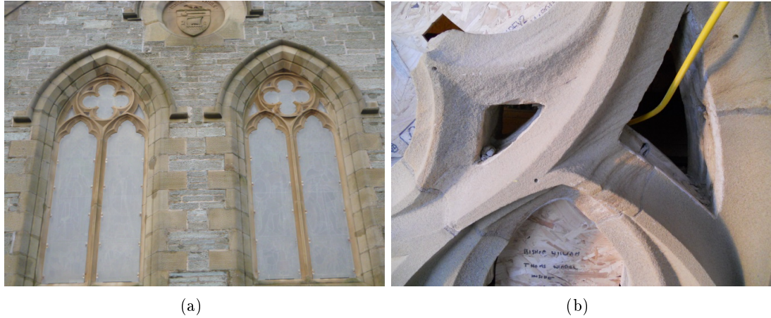
Figure 5.1: Image of the Lancet windows, Lerwick Town Hall (a) and detail of the deteriorated sandstone (b).
