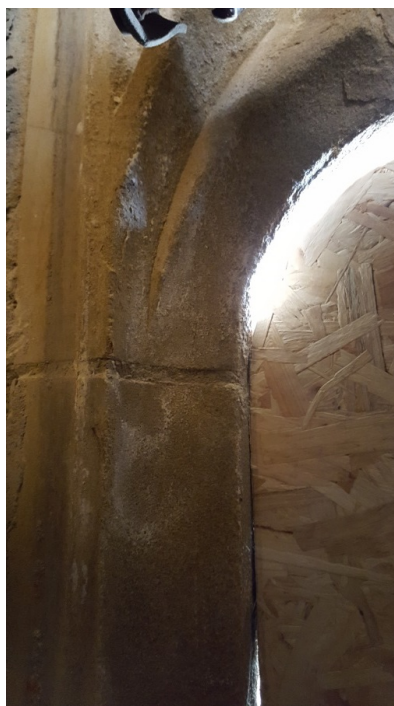
Figure 5.11: Efflorescence on the top of the left side of the left window (from the inside) on the south side of the main all, first floor.
