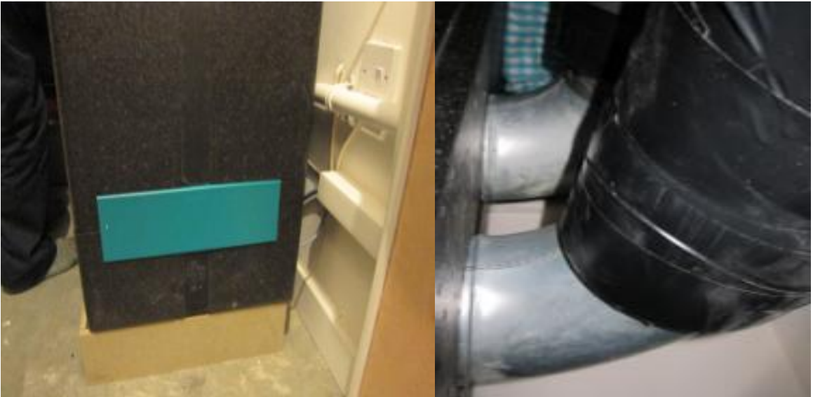
Figure 6.22 – PassiveHouse MVHR Ducting Unit; insulation issue
