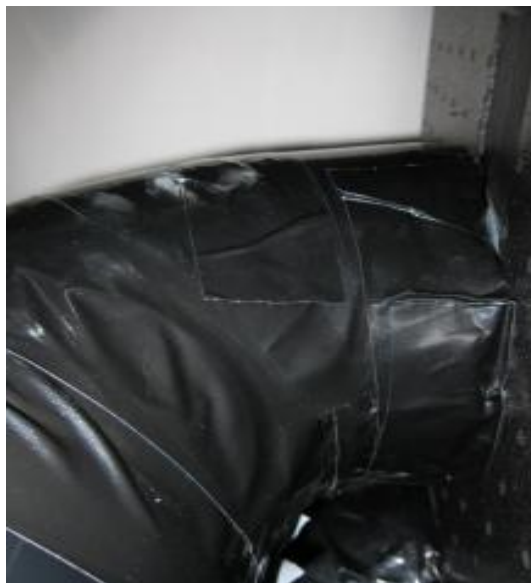
Figure 6.26 – Remedial work to MVHR ducting. Further improvements required so that PassiveHouse standards are met
