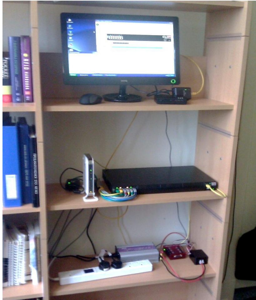
Photograph 5-8 PoE Trial Network Power Components in Situ
