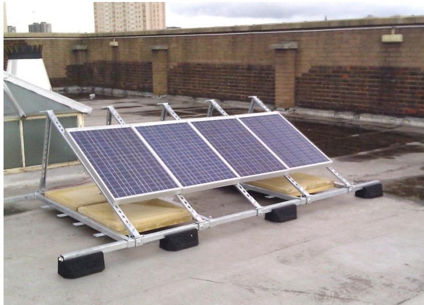
Photograph 5-6 PV Array on Roof of James Weir Building
