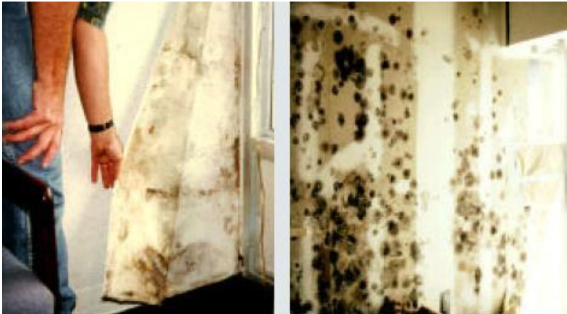
Figure 1.1 Evidence of mould growth behind vinyl wallpaper covering (Lstiburek, 2001).
