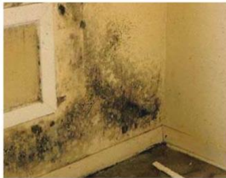
Figure 2.5 Formation of mould as a result of surface condensation (Curtis R, 2007).
