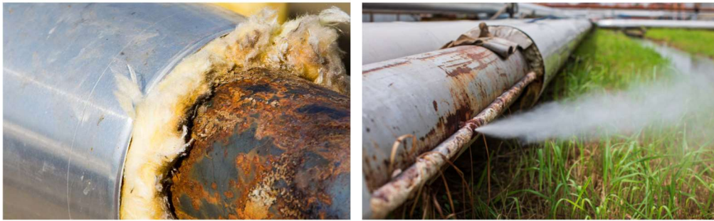
Figure 1-1: Examples of degraded pipework within the oil and gas sector (a) Insulated pipe with cladding removed to show corrosion under insulation (b) Leaked pipework due to corrosion [11].
