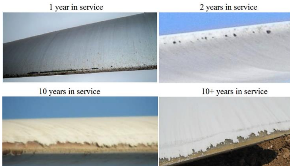
Figure 3-4. Examples of leading edge erosion in the field across a range of years in service. Source: [75]
