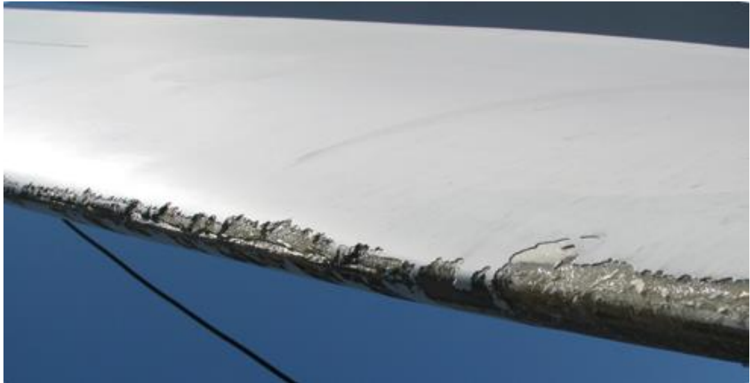
Figure 3-1. Example of leading edge erosion. Source: [63]
