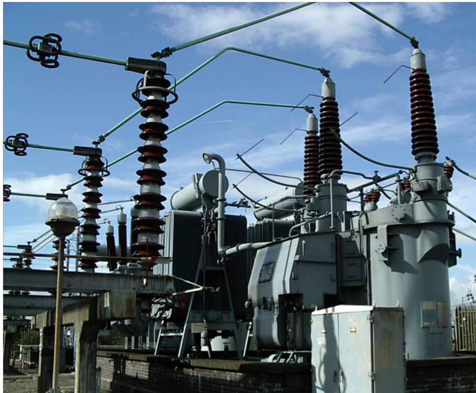
Figure 2.1. 120MVA SGT1 Transformer at Easterhouse, Glasgow, Scotland, which converts 275kV to 33kV (courtesy of V. Catterson, University of Strathclyde)
