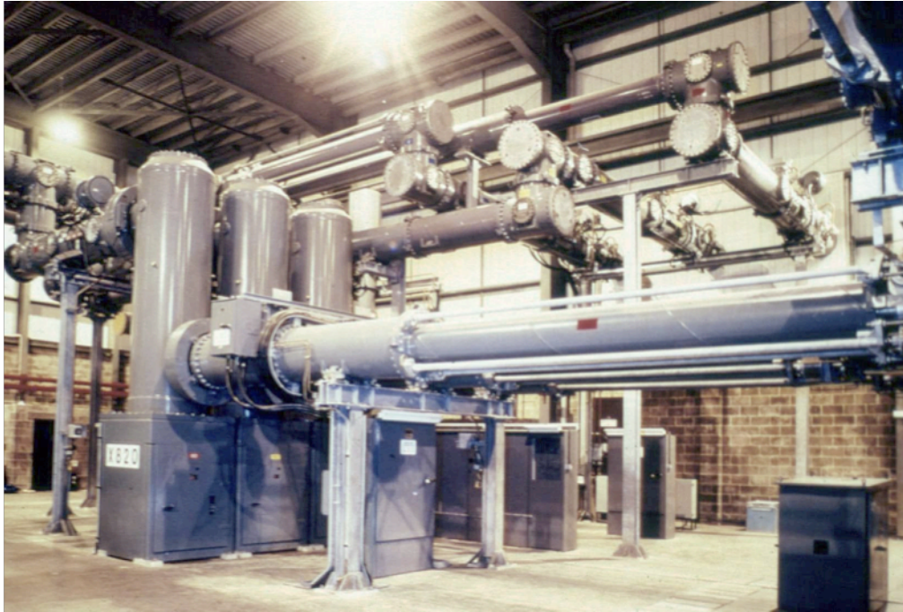
Figure 2.3. 400 kV Gas insulated substation at Torness nuclear generation station
