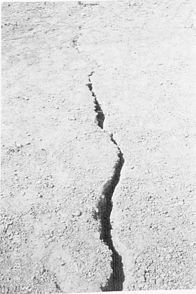
Plate 6.1 : Crack Appearing on the Kuala Perlis South Trial Embankment
