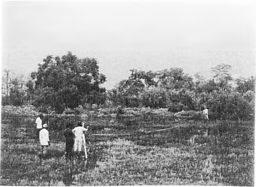
Plate 4.1 : Surveying of the Trial Embankment Site Prior to Main Site Investigation and Instrumentation Works
