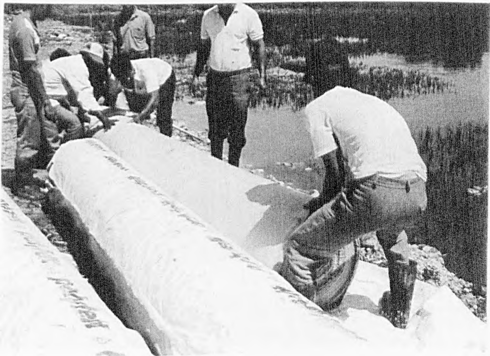
Plate 4.2 : Polyfelt Geotextile TS600 used as a Separator Layer on the Trial Embankment
