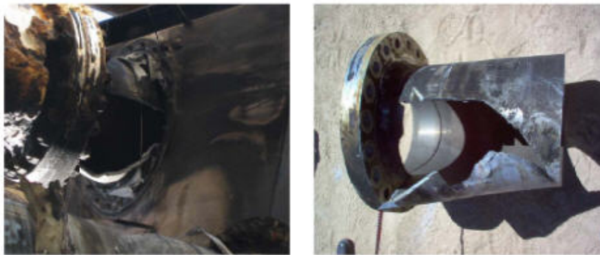
Figure 2.7: Inlet nozzle fatigue due to mercury. Taken from Ref.[67].
