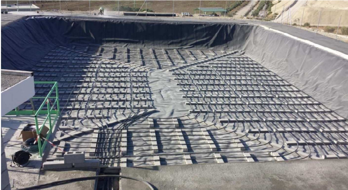
FIGURE 2.18. Heat exchanger (1200 m in length) in the Granada, Spain, distributed in six independent spirals of 200 m each. Fixation of the heat exchanger pipes was done by the use of concrete bricks [27].
