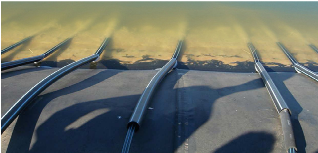
FIGURE 2.20. Heat extraction tubes with insulation and outer tubes [26].
