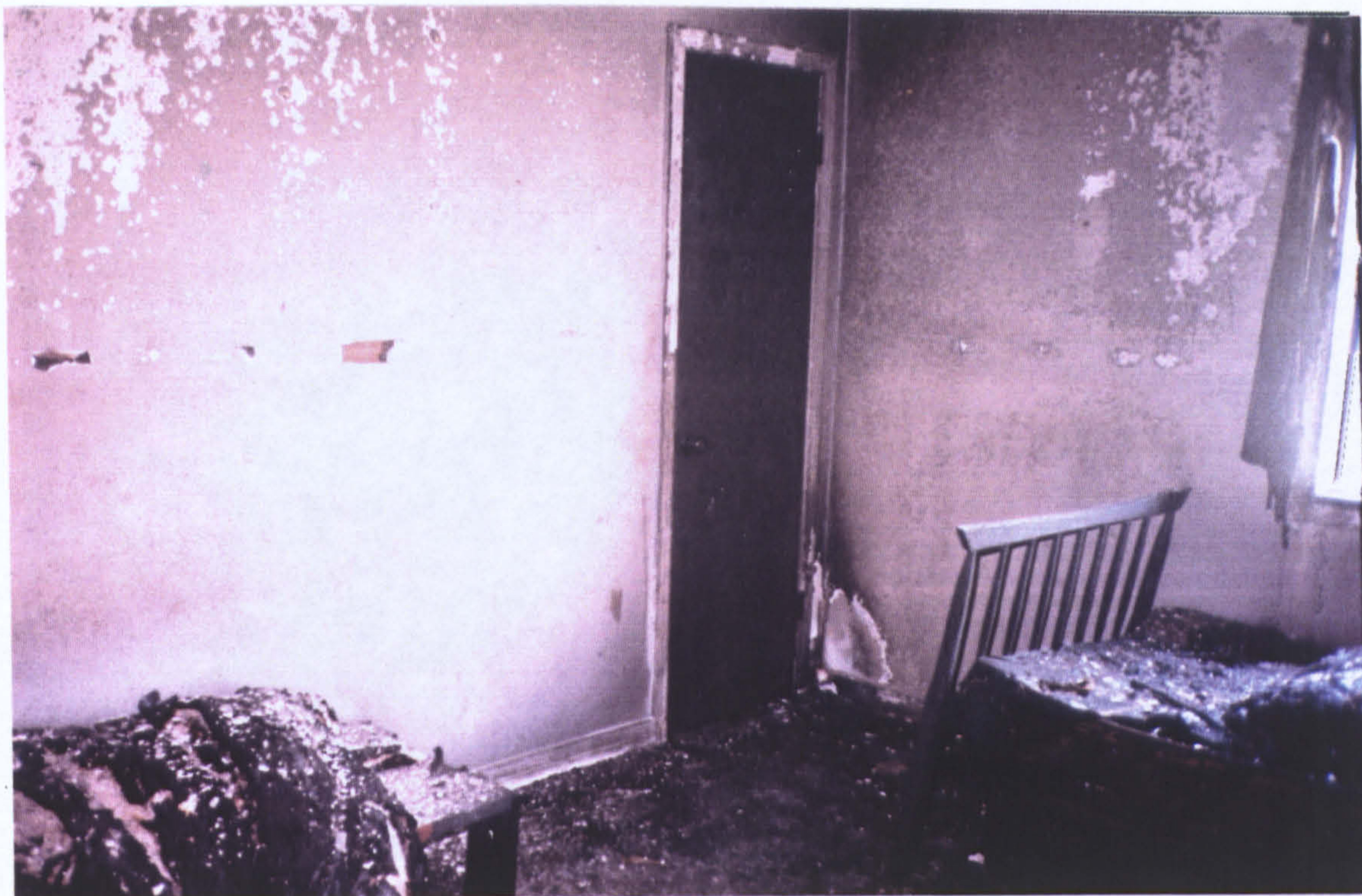
Fig. A3.10.4.10: Results of the same room test (B3) where ~2litres of camping fuel was poured in a random pattern across a furnished, carpeted room, showing an isolated burn in the corner where some fuel was splashed.
