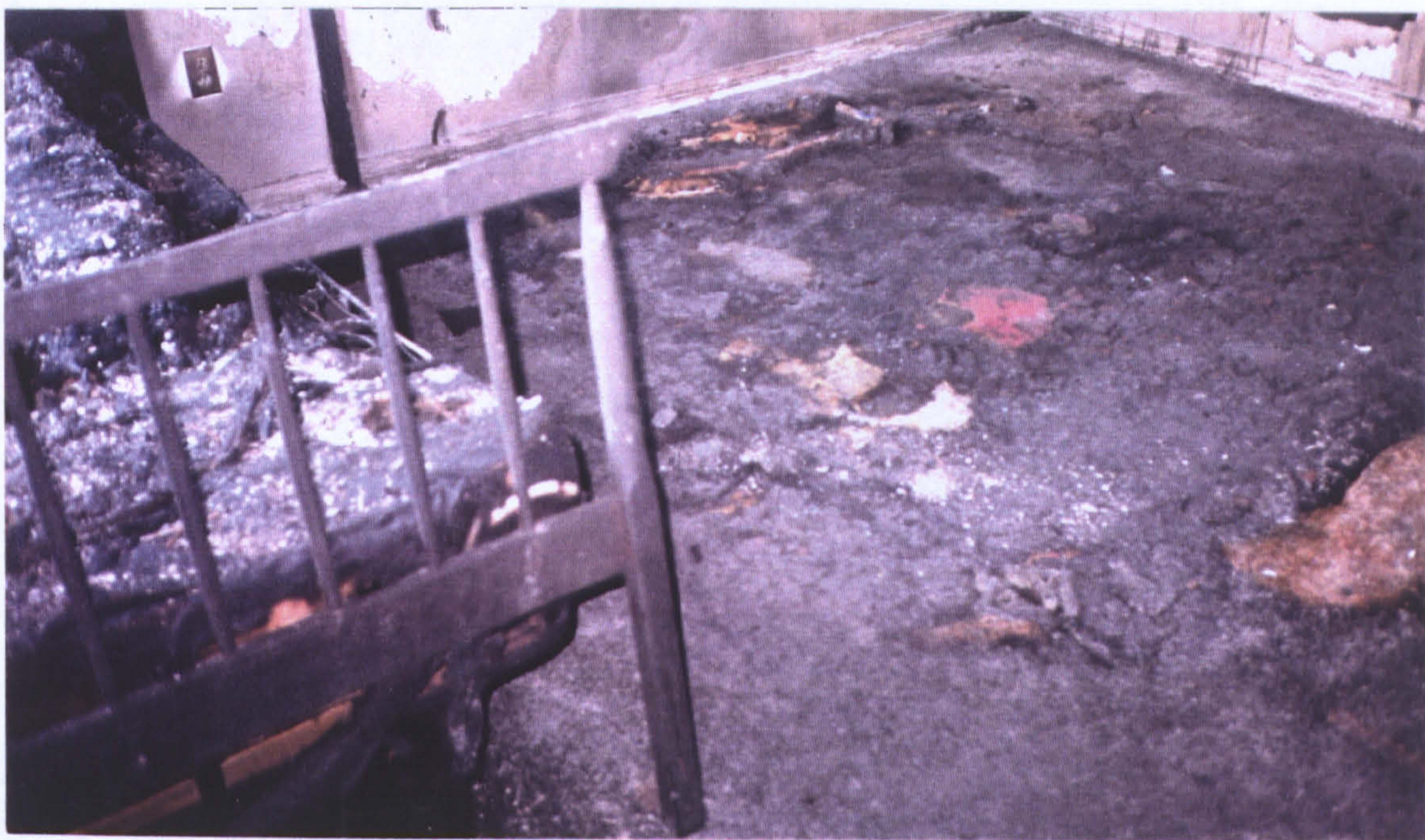
Fig.A3.10.4.8: Results of room test (B3) where ~2litres of camping fuel was poured in a random pattern across a furnished, carpeted room and ignited 40s after pouring was completed. Resulting fire was allowed to grow to flashover and then extinguished. Furniture has been removed to reveal damage to carpet. Extensive surface charring not associated with pour pattern is visible. Some localized deeper damage is visible in the centre of the room. Portions of that penetration co-incide with the pour pattern.
