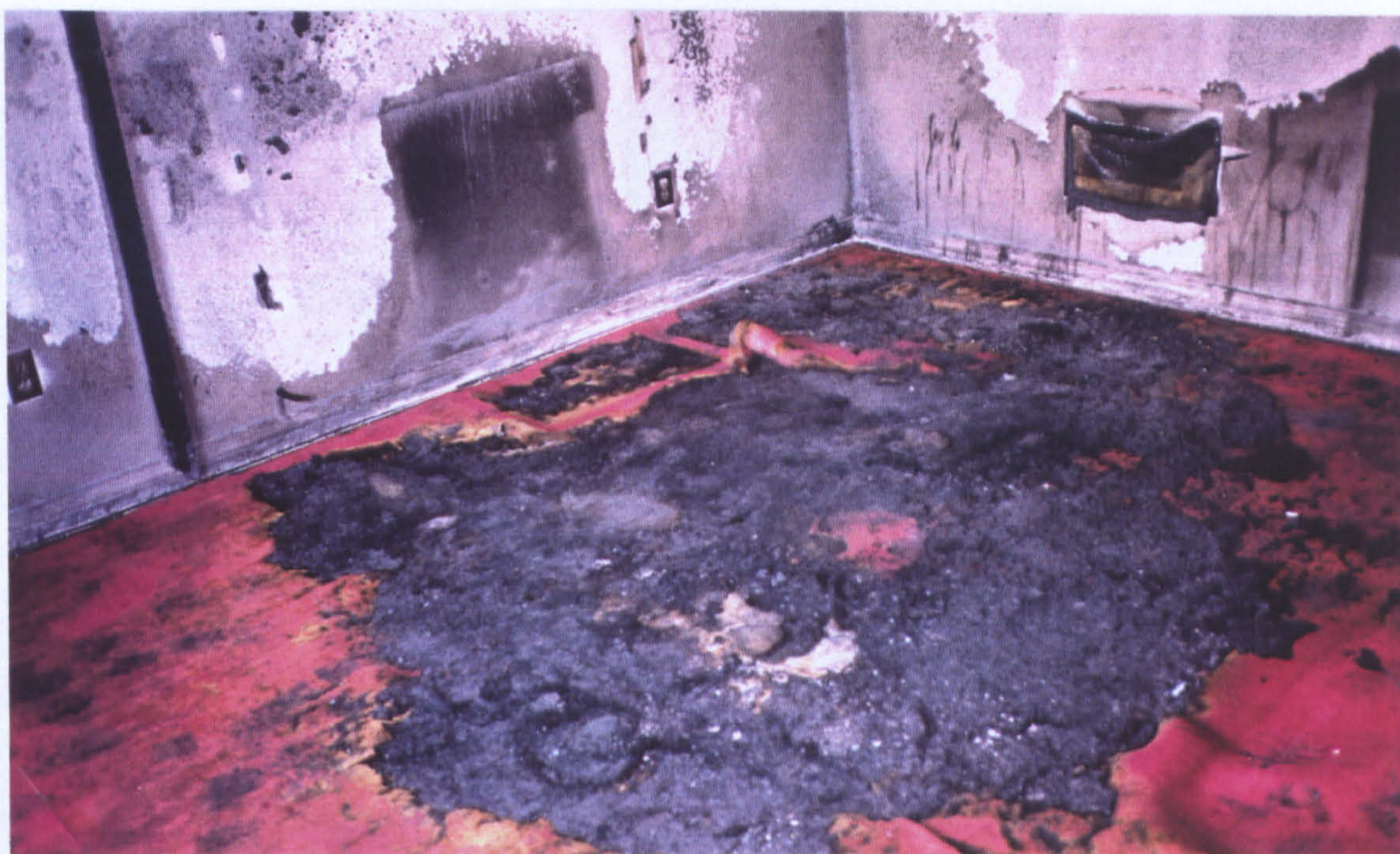
Fig. A3.10.4.9: Results of room test (B3) where ~2litres of camping fuel was poured in a random pattern across a furnished, carpeted room. The carpet has been removed to exposed the damage to the underlying urethane pad (with vapour-barrier). The circular pattern in the centre of the room and the rectangular area parallel to the far wall co-incide with the pour pattern. The areas involved are much wider than the pour pattern (on a 6–7mm deep nylon pile carpet). There are also undamaged areas where fuel was known to have been splashed.
