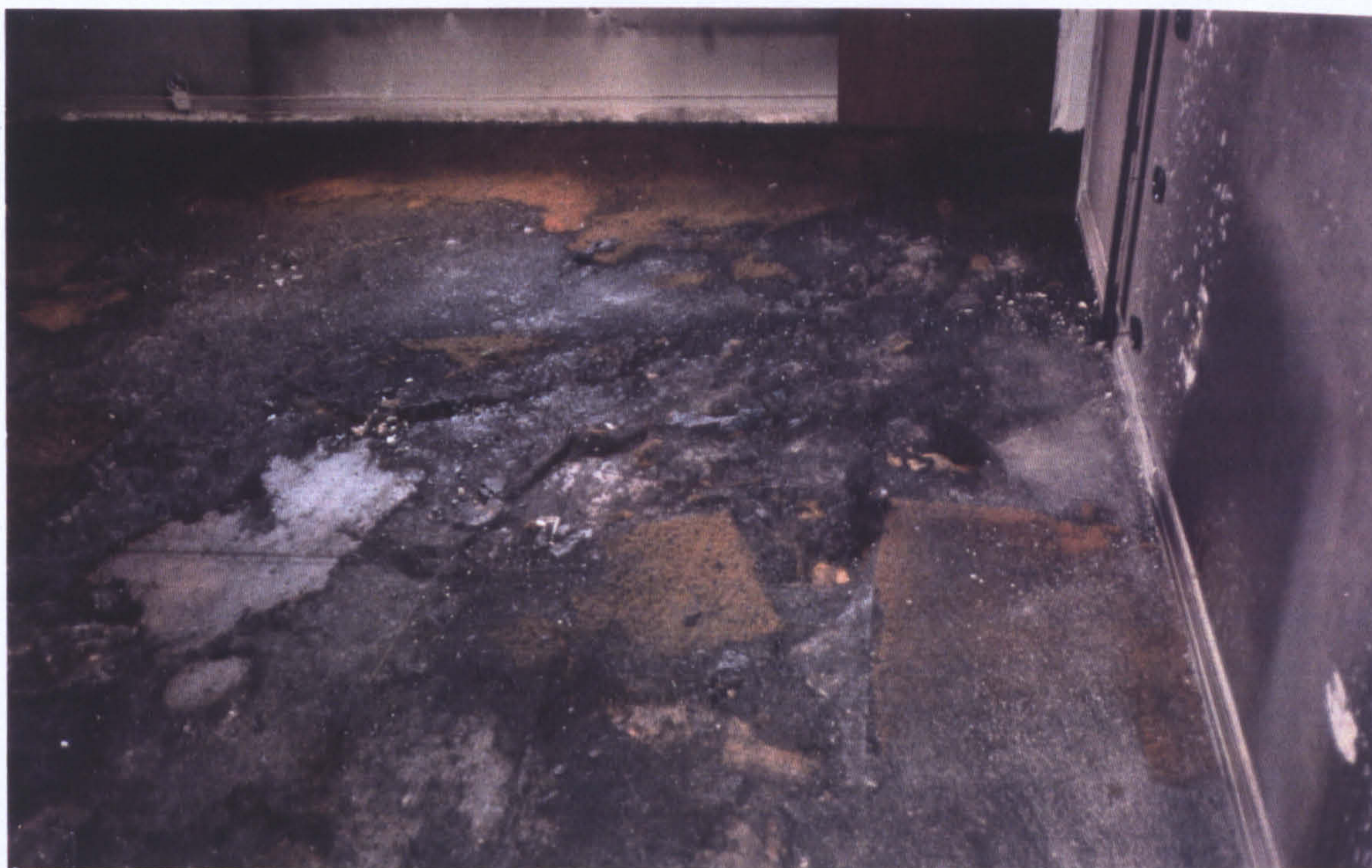
Fig. A3.10.4.13: Another view of the same room showing heavily damaged areas of carpet that co-incide with the location of the fuel pour, but not size (area).
