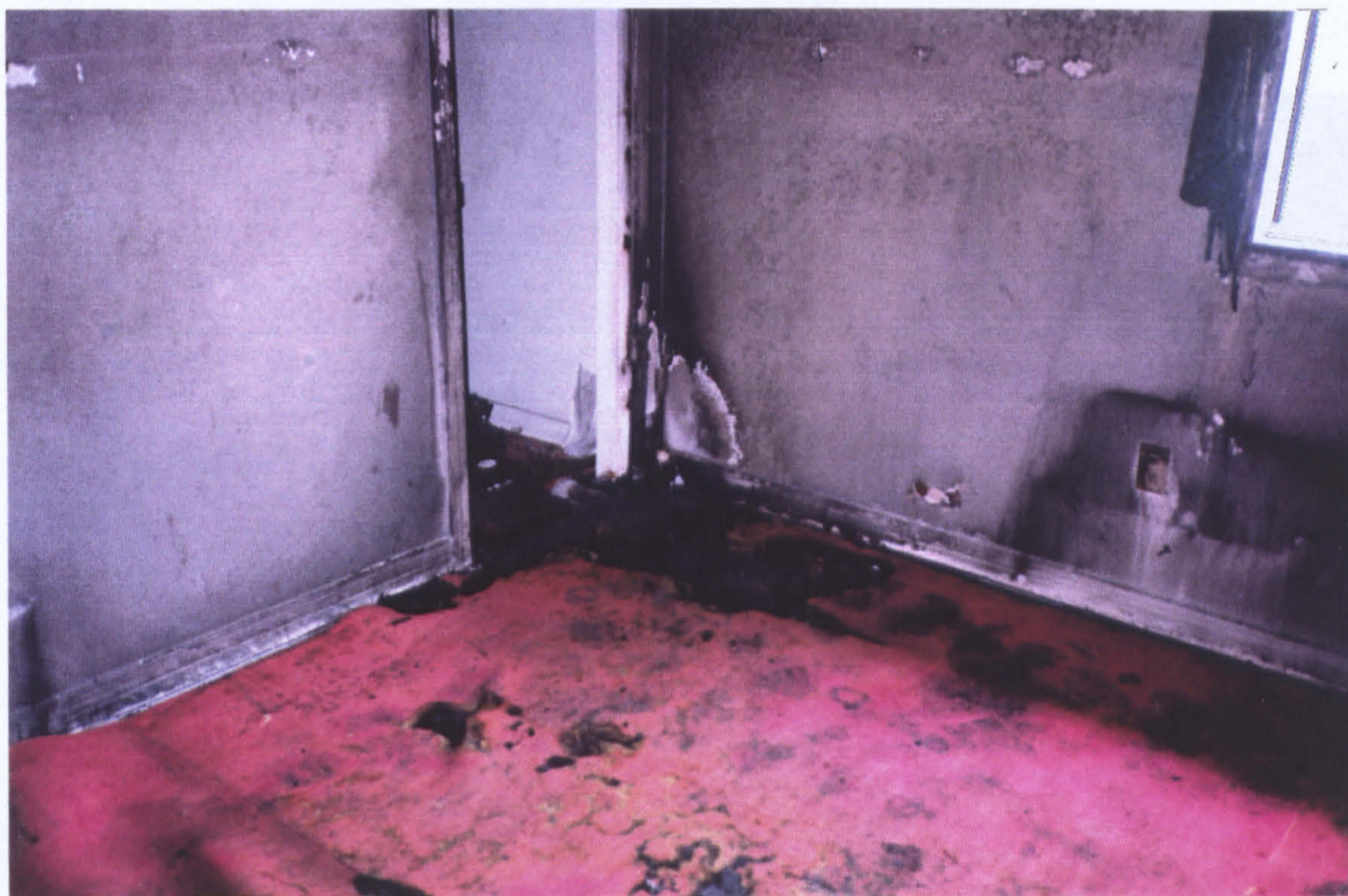
Fig. A3.10.4.11: Results of the same room test (B3) showing the corresponding area of damage to the underlying carpet pad. The location of the pour pattern is detectable, but the size is larger than the original pool.
