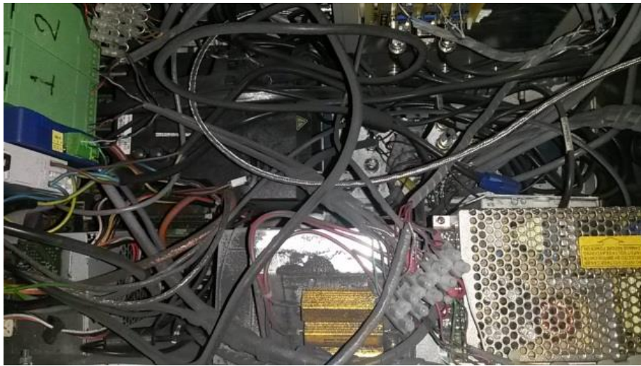
Figure 22: Large volume of dust inside enclosure
