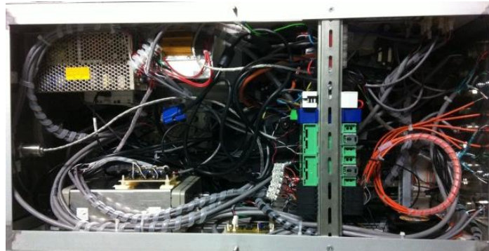
Figure 15: Inside main enclosure
