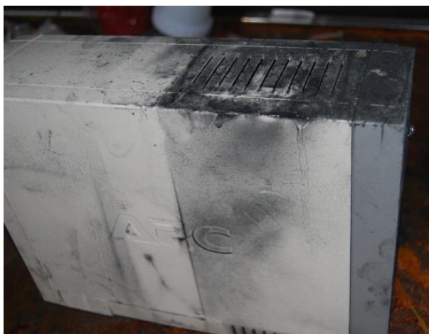
Figure 23: Failed UPS due to excessive dust
