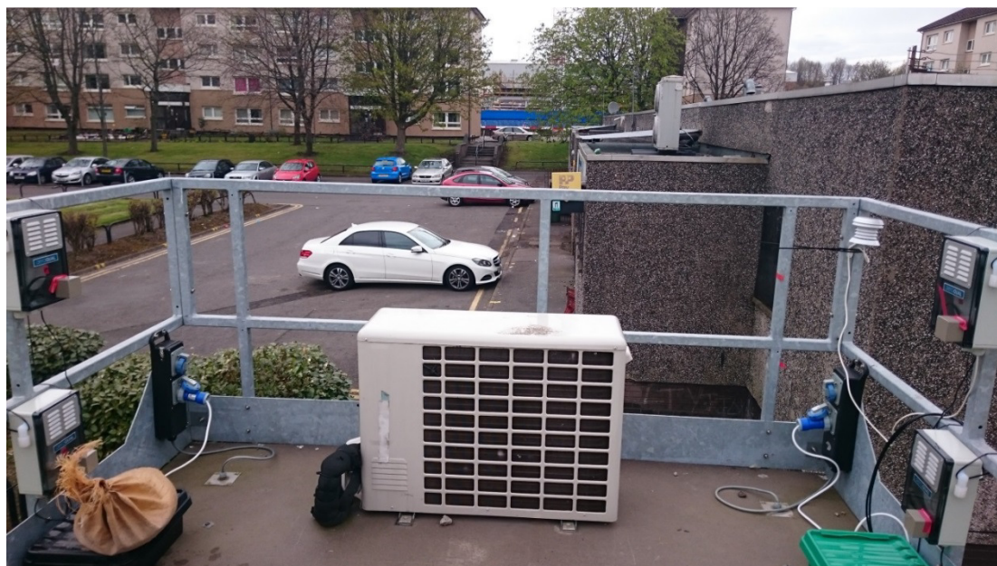
Figure S1: Deployment of Aeroqual monitors on the roof of Glasgow Townhead AURN station. The monitors were deployed within ventilated waterproof enclosures provided by Aeroqual attached to the galvanised steel safety railings surrounding the roof of the AURN monitoring cabin.
