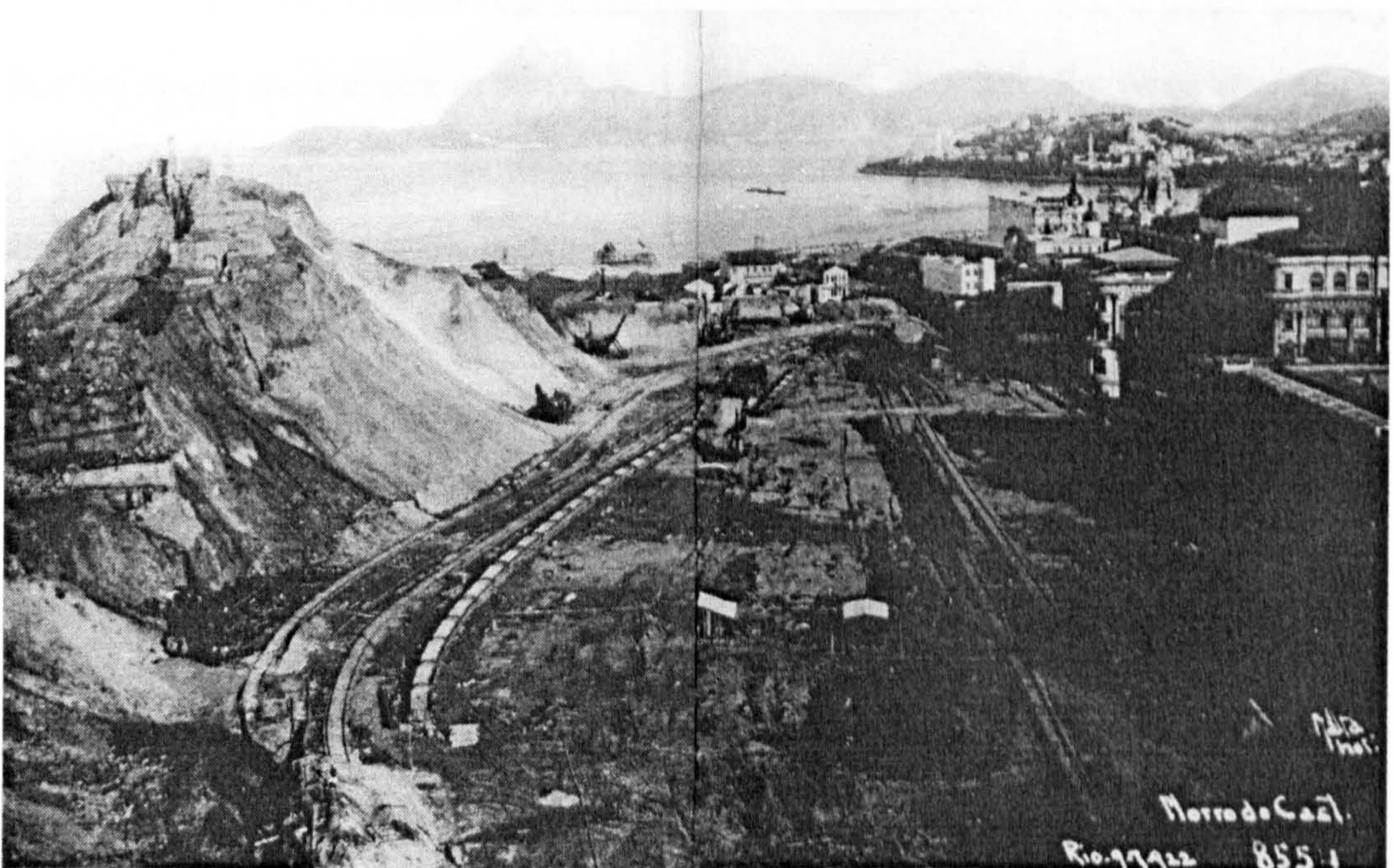
Figure 5.3: The dismantle of the Castelo Hill in the center of Rio de Janeiro. Photograph by Augusto Malta, 1922. "Album de fotografias do Castelo," 1922 (Nonato and Santos 2000)
