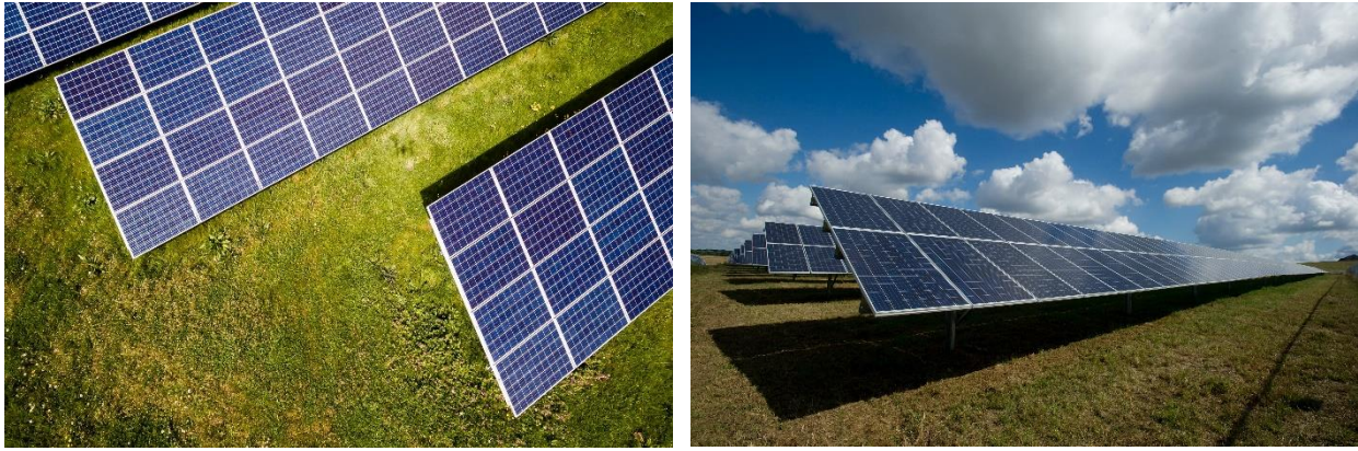
Figure 2.1. PVPS as deployed in Germany (Photo by Andreas Gücklhorn on Unsplash) and in the United States (Photo by American Public Power Association on Unsplash).
