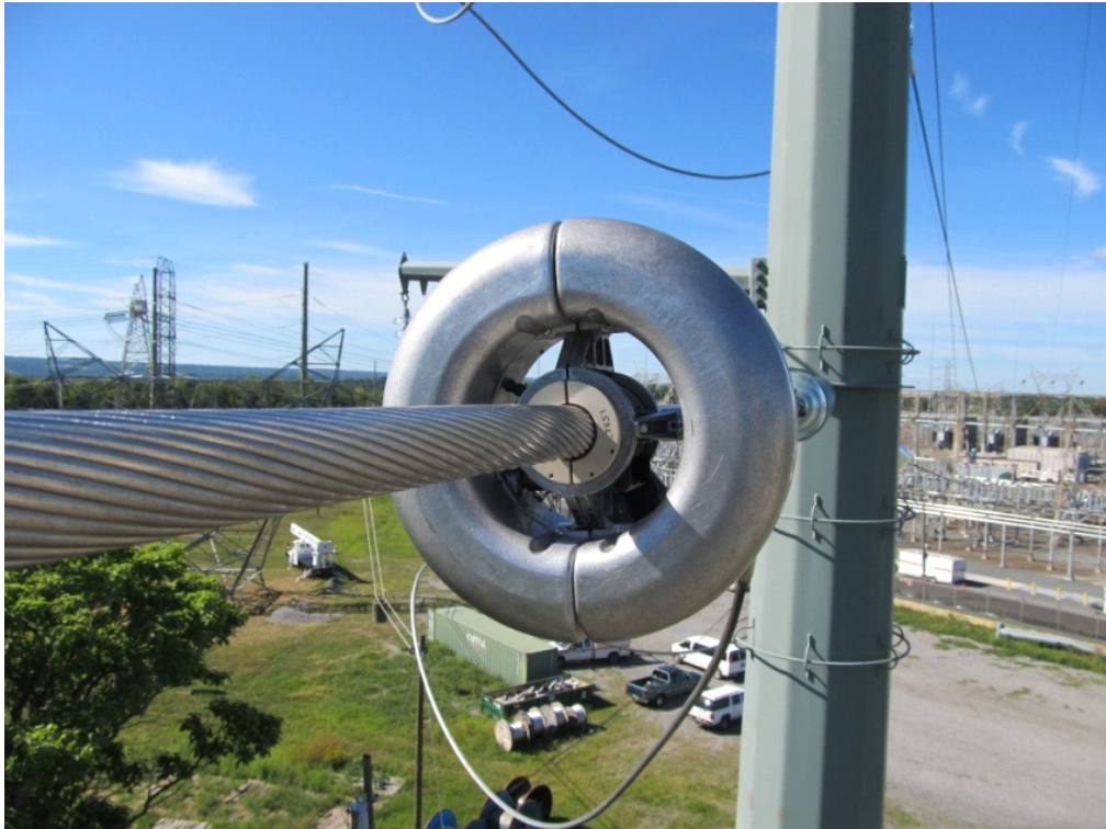
Figure 2.13: An installed power donut line monitor [38] © Underground Systems Inc 2016.
