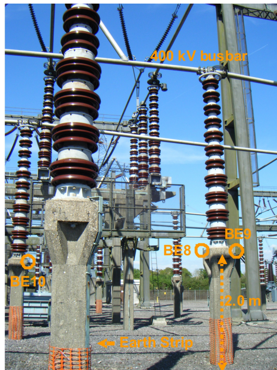
Figure 3.13: Measurement points around the concrete support posts of 400 kV busbars in Bolney substation.
