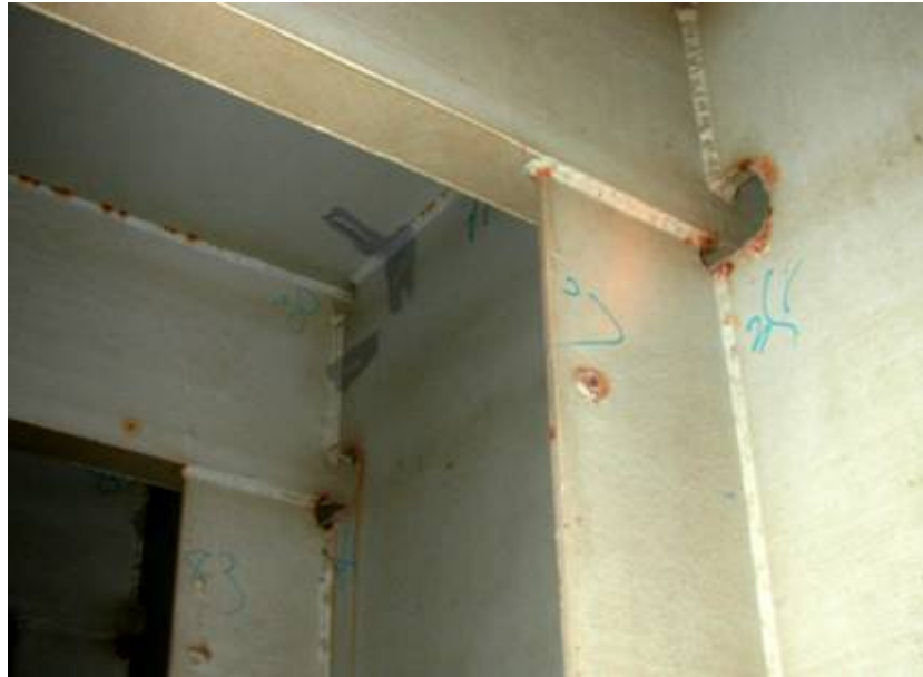
Figure 8.67 Stress fatigue crack found at cut-outs of Bulk carriers ( http://www.amteccorrosion.co.uk/papers/coatingfailuresguide.html )
