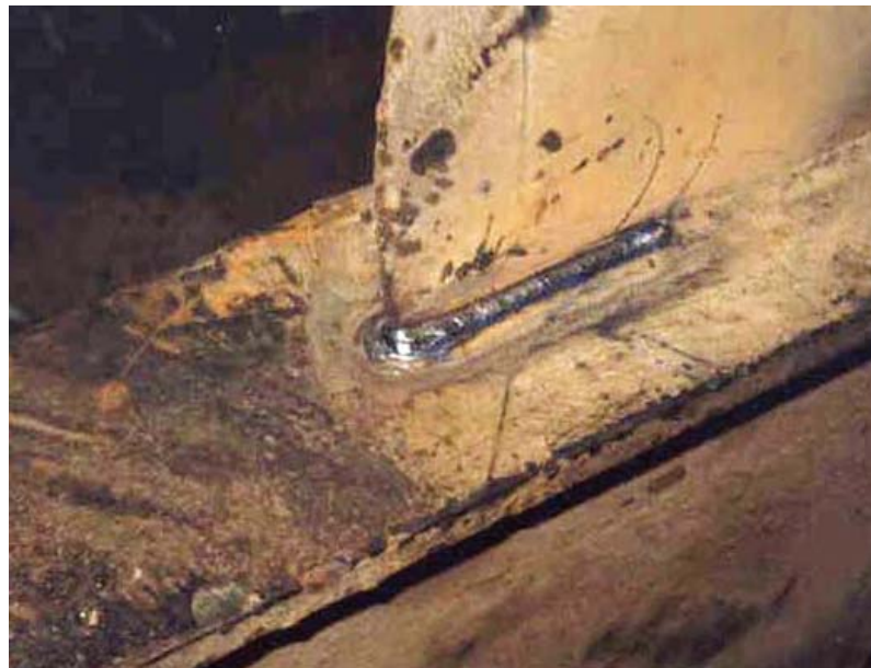
Figure 2.5 Fatigue crack at the bracket end of longitudinal stiffener (R.V. Guchisky, S.V. Petinov, 2011)
