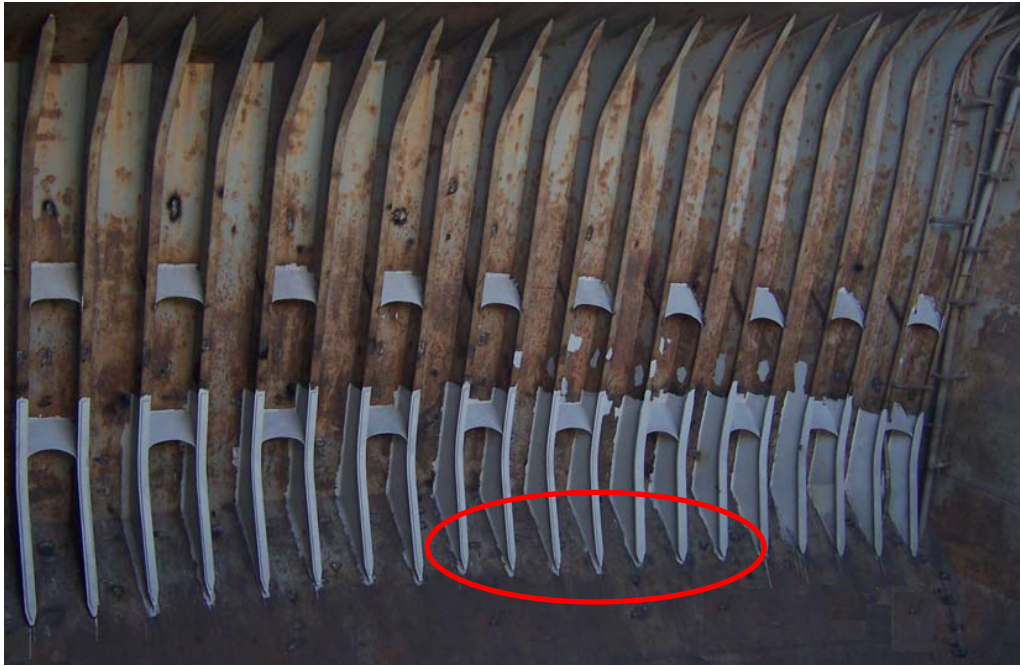
Figure 8.53 Structural reinforcement using Tripping Brackets (LR, Thickness Measurement and close-up survey guidance Part1, 2012, P43)
