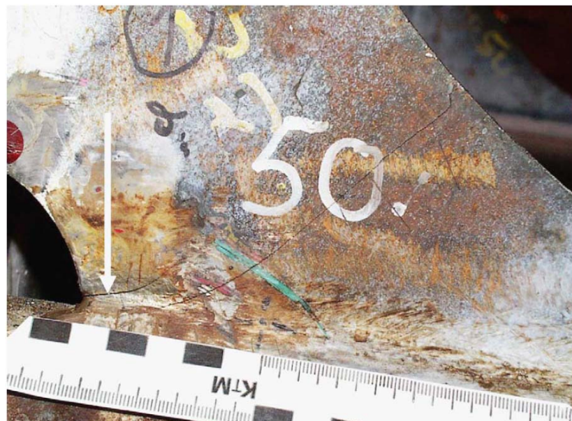
Figure 2.6 Fatigue cracks growth along the bracket plate (I. Lotsberg, En Landet, 2005)
