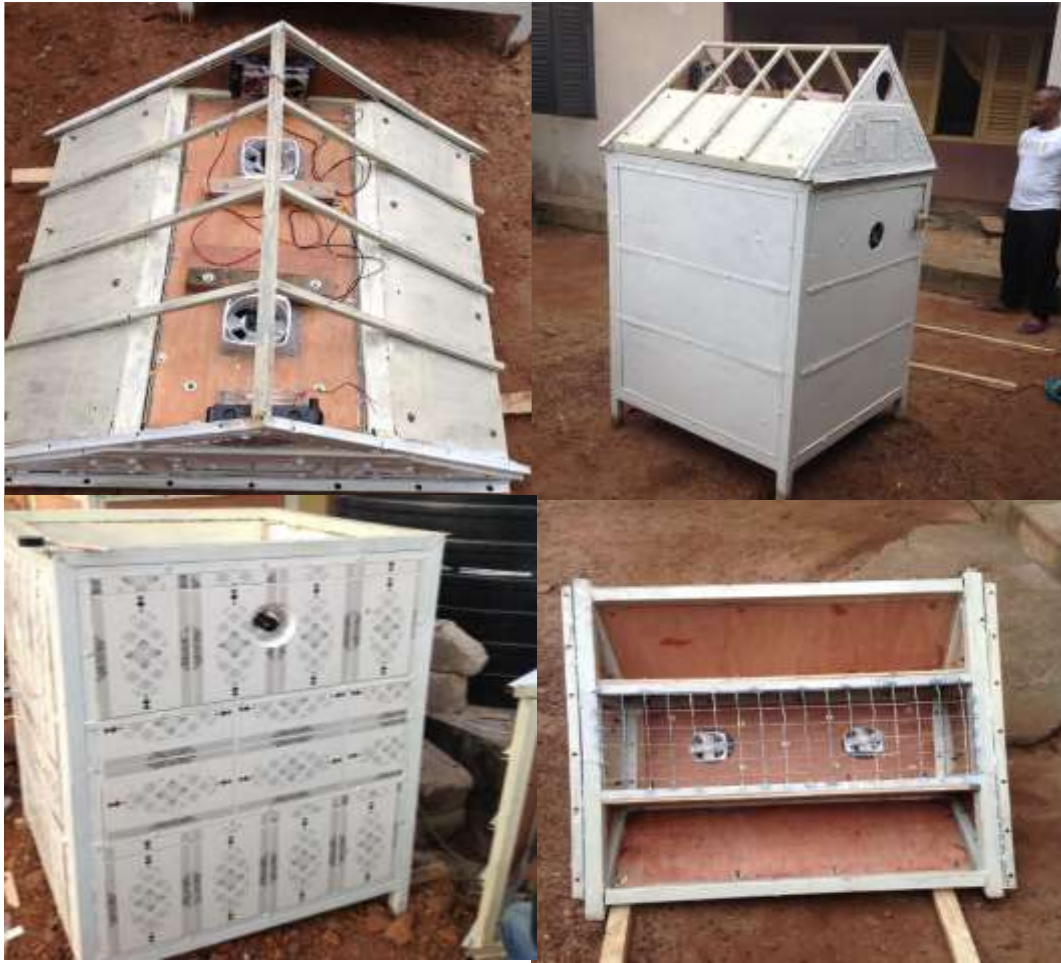
Figure 5. 27 Roof structure under construction showing details of Insulation and air inlet plenum in the proposed experimental cell
