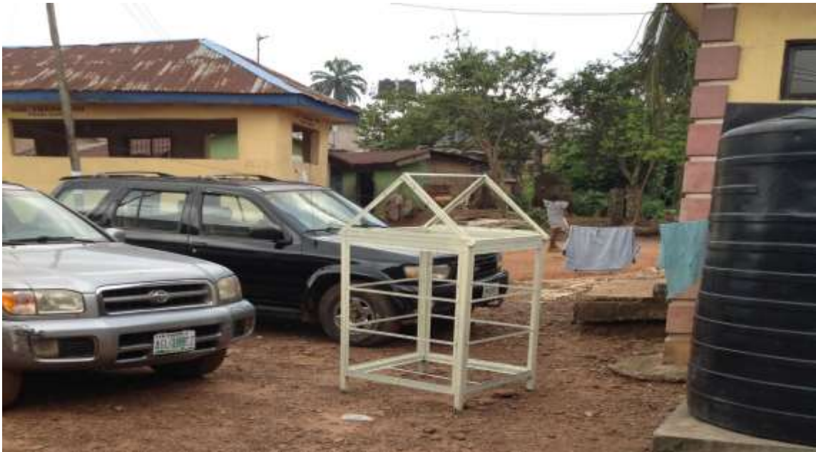
Figure 5. 11 Picture showing a finished metal frame for one of the experimental test cells
