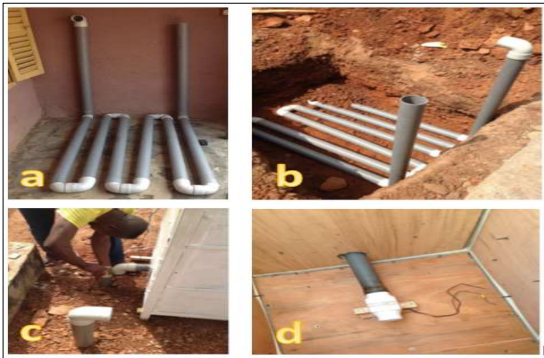
Figure 5. 37 The PVC pipes held in place before installation (a). 1.4x1.4x1m depth pit to receive the underground pipes and (b). Coupling of 50mm diameter PVC pipe to the experimental cell (c) and in-blower fans connected to PVC inlet pipe from underground pipes before floor finish (d)
