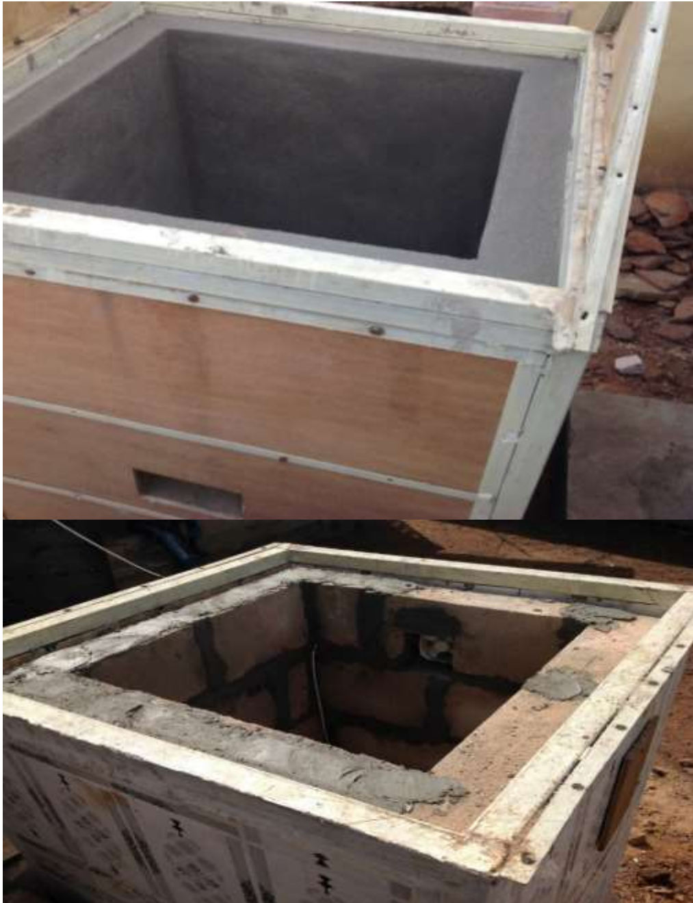
Figure 5. 15 Pictorial View of PCS 1 and PCS 2 under construction. Walls in PCS 2 are finished in heavy thermal mass for coolth storage U-Value 0.39 W/m 2 K
