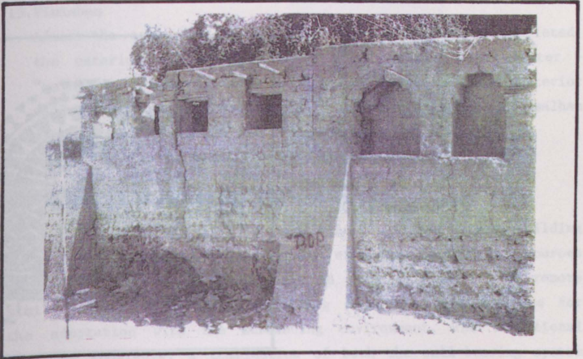
Fig. 64 : A photograph showing the buttresses constructed to support a cracked wall (15).
