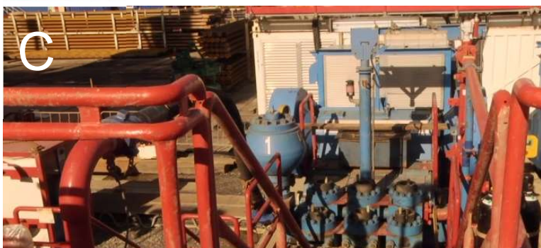
Figure 4.12.C: A view down the stairs from the mud tanks to one of the three mud pumps at the PNR site. These mud pumps provide the hydraulic pressure for the rotation and turning of the drill bit at the bottom of the borehole.
