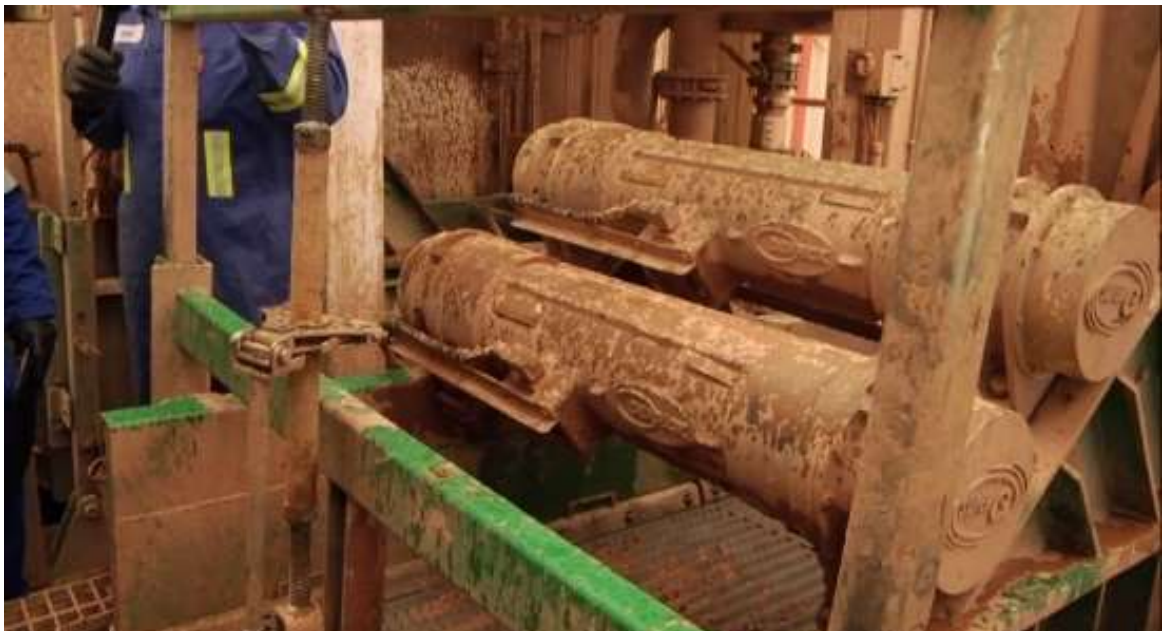
Figure 5.5. A photograph of the shale shaker present at Preston New Road Unconventional oil and gas development site. The two tubular features are vibrating motors which power the vibratory action of the shale shaker.
