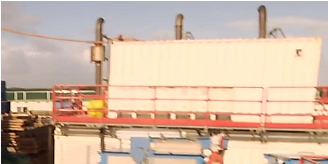
Figure 4.10. A photograph with the three diesel engines displayed. The diesel engines are C12's housed within shipping containers. The exhaust from the engines are extended vertically from the container 3 meters in the air.
