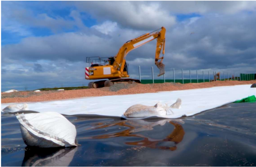
Figure 4.8.A: A Backhoe excavator moving aggregate over two Geotextile Layers. The black layer is a HDPE liner laid down to protect against surface water intrusion whilst the white layer is a protective layer to prevent damage to the HDPE liner.
