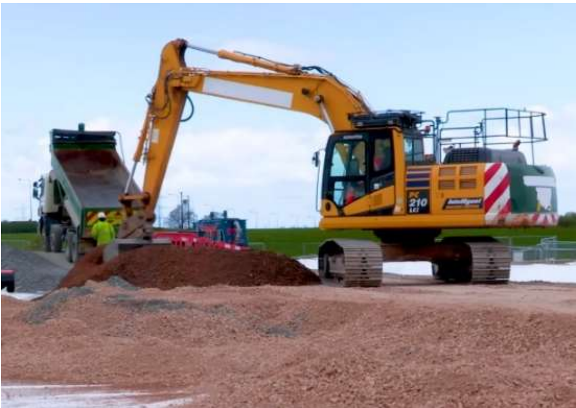
Figure 5.3. Showing a tipper truck and a 10-tonne excavator working gravel on the Preston New Road Unconventional oil and gas development site. The limestone in this case came from a local source of Devensian Limestone which had been pre-sized. However, some of the gravel was screened onsite for specific uses such as screed materials.
