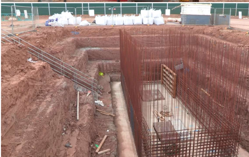
Figure 4.8.C: A Figure showing the construction of the concrete cell where the BOP and other safety equipment will be located. The excavation will later be filled with concrete.
