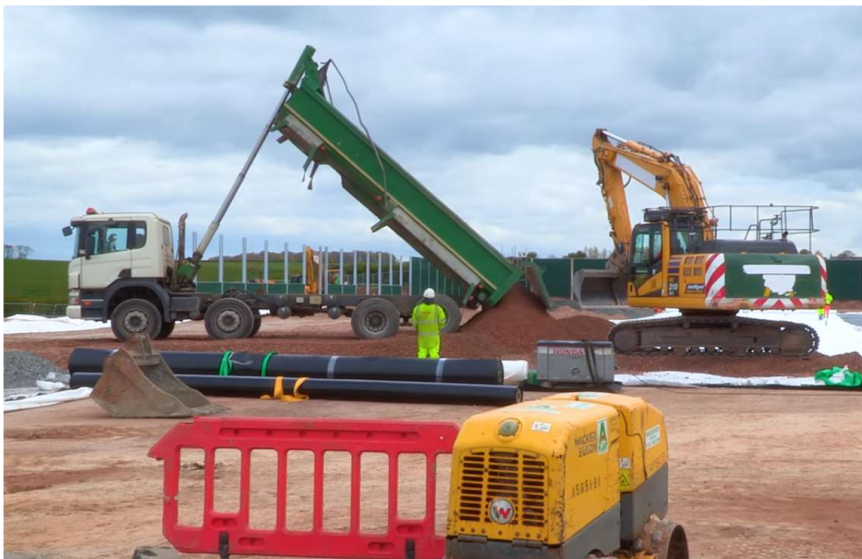
Figure 4.8.B: A Backhoe excavator moving aggregate away from a 20-tonne tipper truck. In the background right is the excavator, whilst in the foreground is a small diesel engine providing electricity to a compressor and lighting (out of frame).
