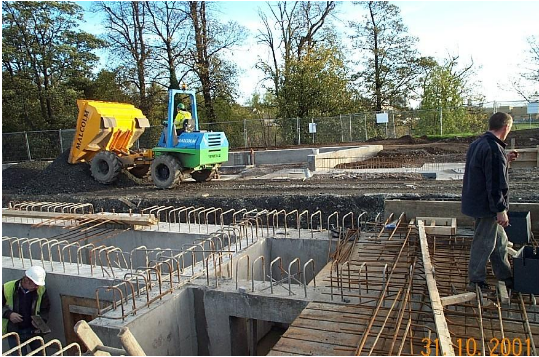
Figure 3.10: Picture of Drumchapel air culvert under construction (Glasgow City Council Development and Regeneration Services 2001).
