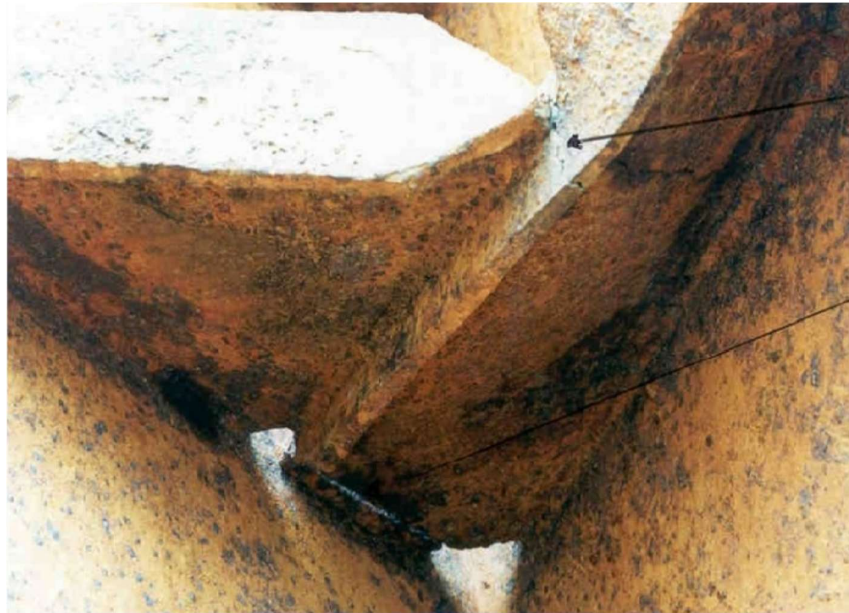
Figure 2-1 Fatigue failure of welded components (Shen, 2015)
