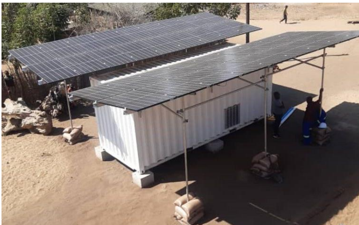
Figure 41 Installed microgrid at Mthembanji
