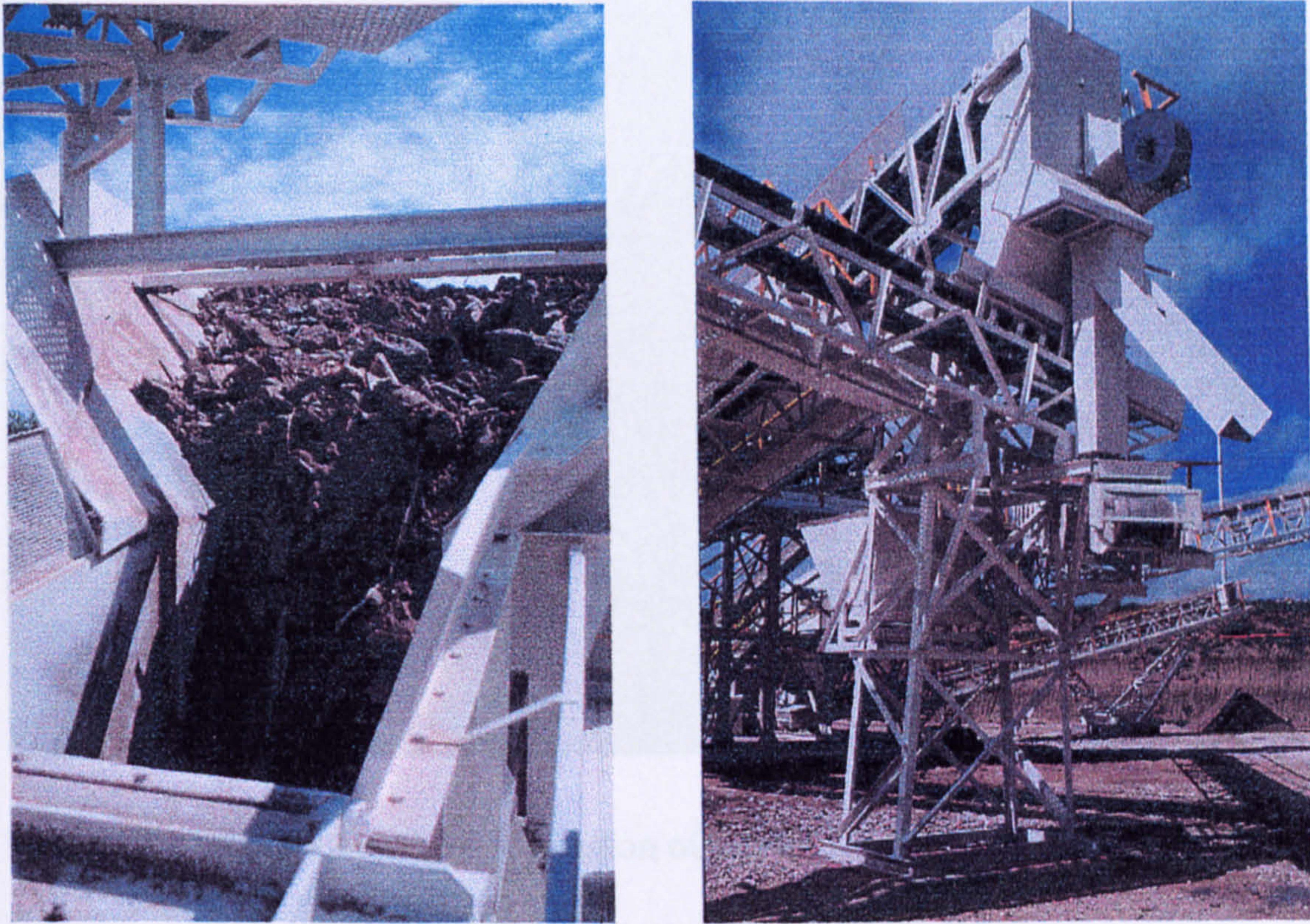
Fig. 3.4 Loading hopper and crossing node for shunting of the material.
