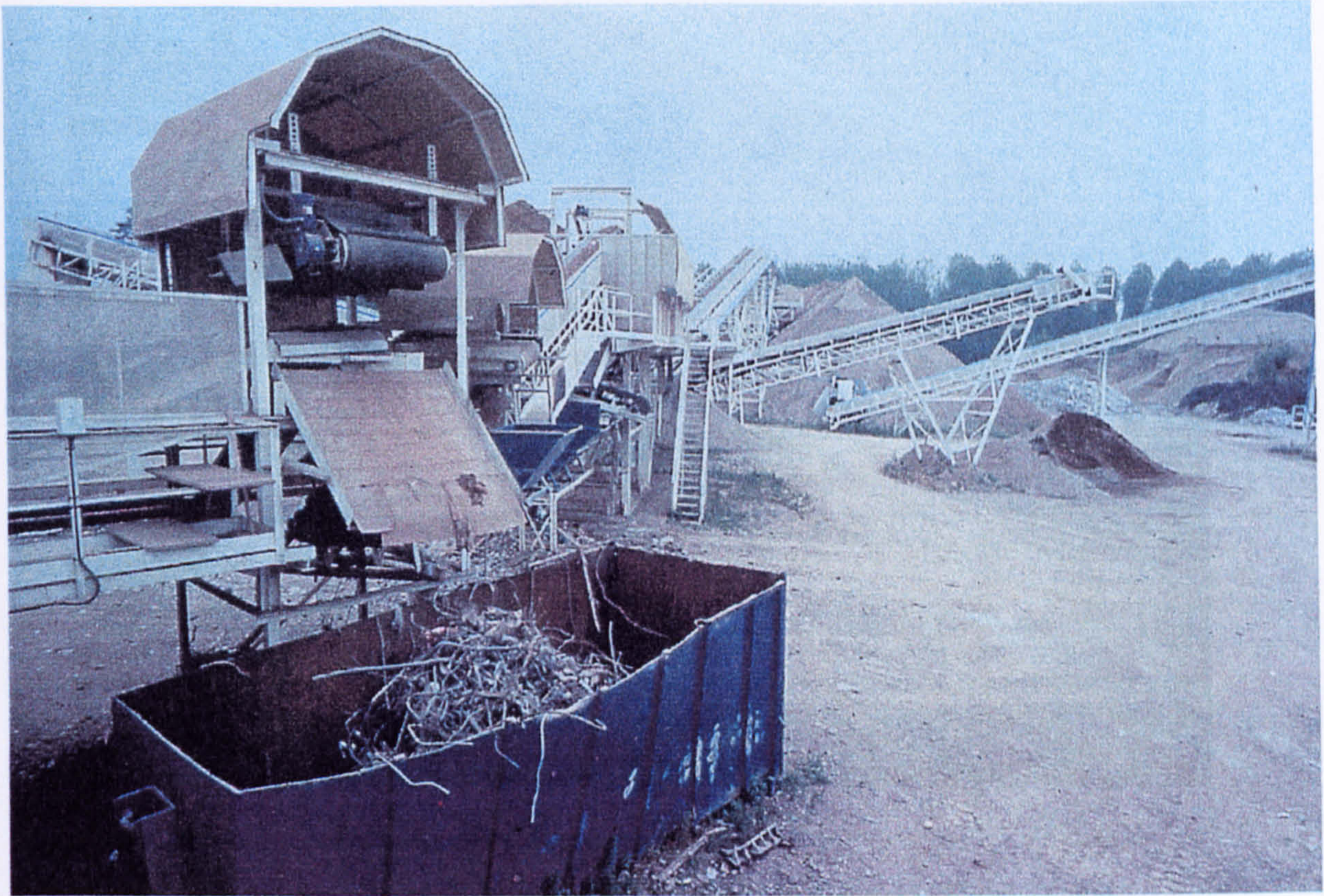
Fig. 3.5 Electric magnet for separation of steel.
