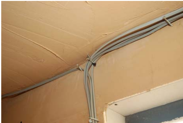
Figure 43 – Cables fixed with screws and cable ties above and to the side of the compartment's entrance doorway.
