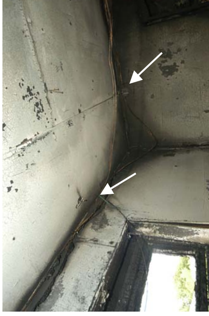
Figure 666 - Post-fire view of the ceiling above the fire's dominant plume. The left arrow details the arcing damage location of circuit 4 (exhibit 101). The right arrow details exhibit 098 (circuit 1).
