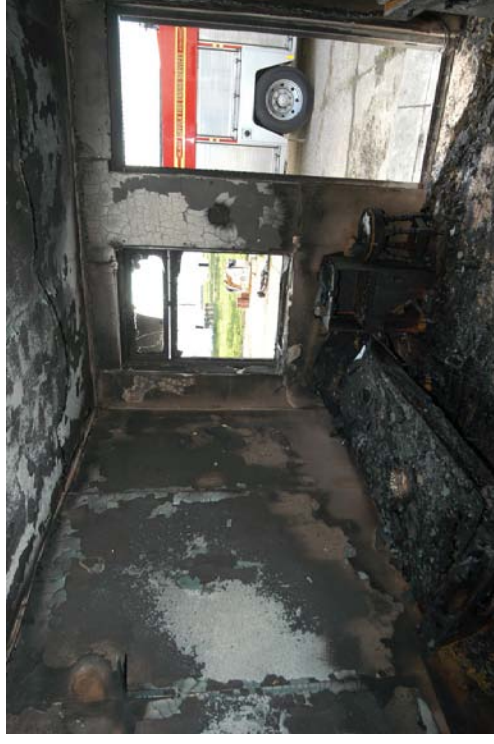
Figure 293 - Post-fire image of the compartment viewing the entrance door.
