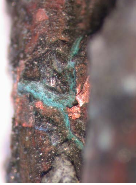
Figure 298 - 40x magnification of the bottom conductor damage detailed in figure 295.
