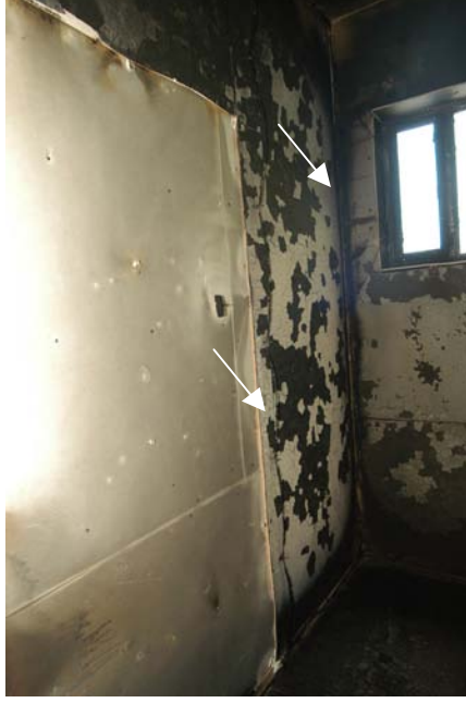
Figure 628 - Post-fire view of the ceiling above the area of origin. The left arrow was the arcing location of circuit 4 and the right arrow was the location on circuit 1.
