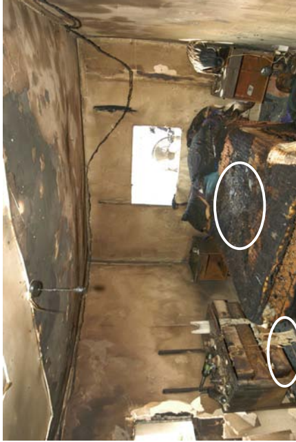
Figure 63 - Post-fire photograph of the view above. The white ovals indicate the fire's areas of origin.
