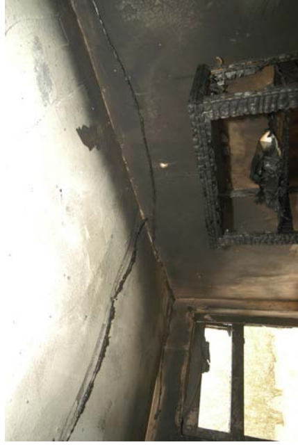
Figure 483 – Post-fire image of circuits 1 and 4 on the ceiling above the display unit.
