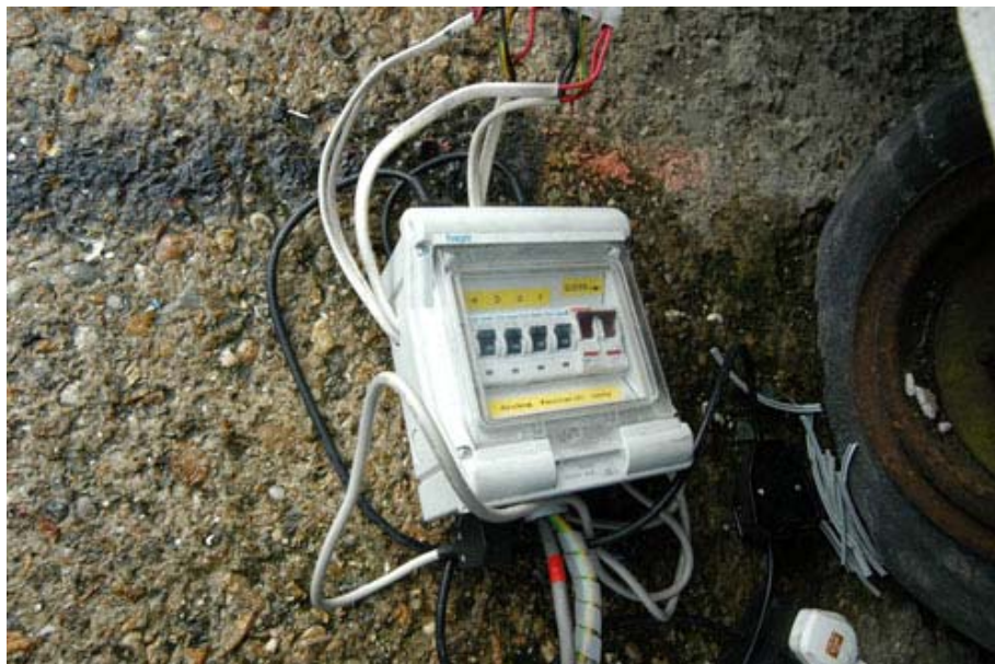
Figure 51 – The portable distribution board constructed to IP 55 ingress protection.
