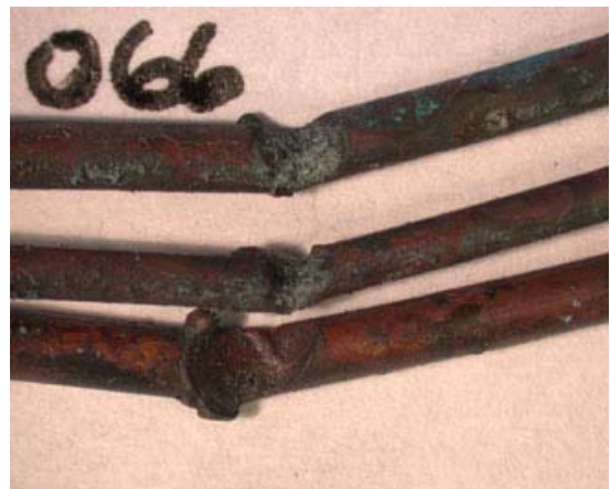
Figure 30 – All three conductors of this cable are affected. The arcing has occurred at a fixing screw. All are notched with beading on the notch edges.
