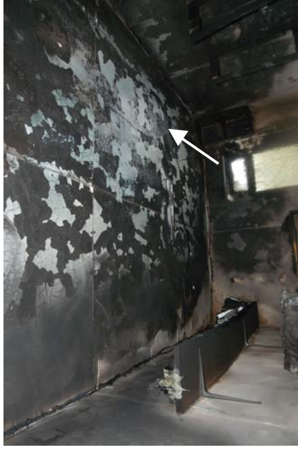
Figure 434 - Post-fire photograph of the compartment with a white arrow indicating the arcing damage location on circuit 4 that was within 0.5m of the wardrobe edge.
