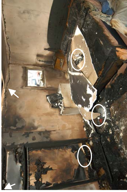
Figure 272 - Post-fire over-view detailing the fire's area of origin. The arrows detail the arcing damage locations to circuit 1 (left of wardrobe) and circuit 4 (above the bed)
