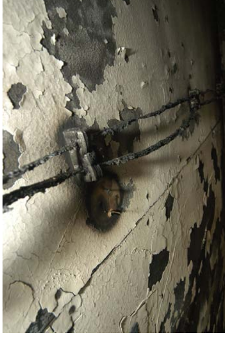
Figure 930 - Close-up post-fire view of the wood blocks used to support the ceiling wiring.
