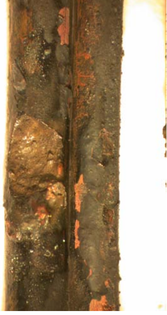
Figure 378 - A notch on one conductor with a bead to the side.
