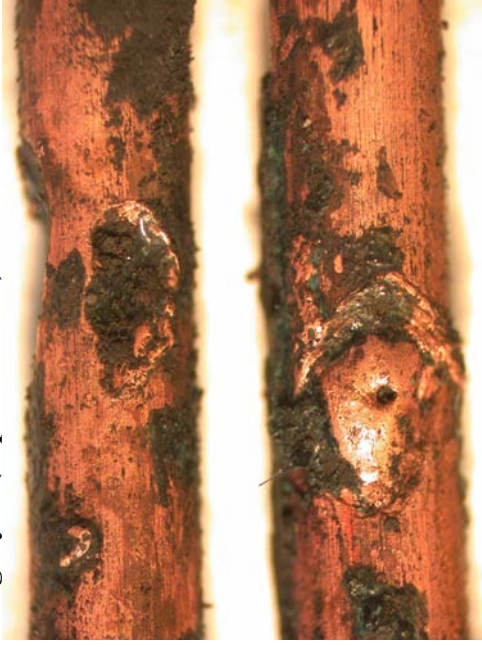
Figure 631 - View of both conductors and the notch damage on the conductors.
