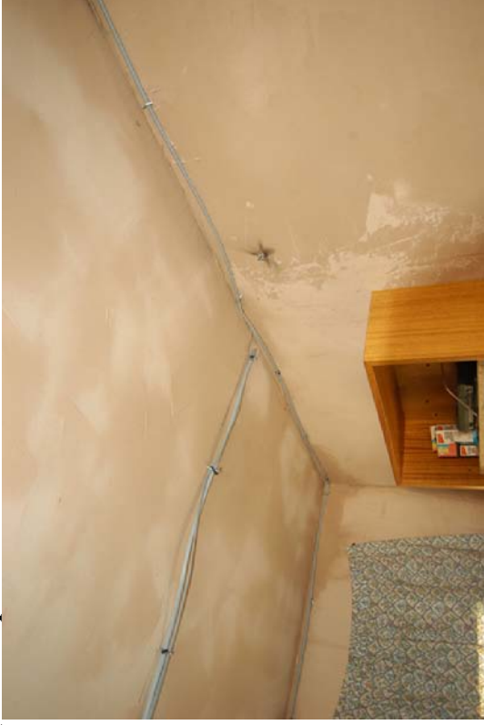
Figure 312 - Pre-fire view of wiring installed on the ceiling.
