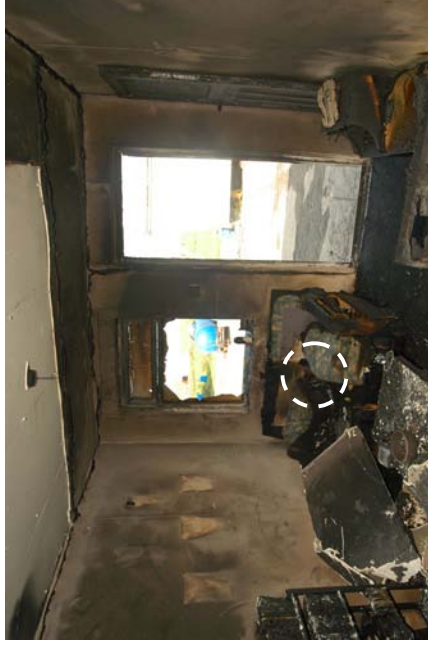
Figure 603 - Post-fire view of the front area of the compartment with the entrance door in the background.
