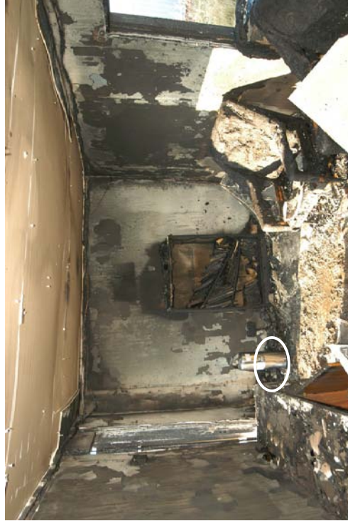
Figure 39 - Post-fire photograph of the view above. The black oval indicates the 3rd area of origin.
