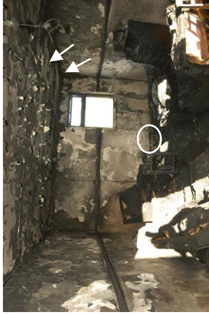
Figure 982 - Post-fire view of the fire scene with the area of origin indicated with a white circle as above. The left arrow is arcing damage to circuit 1 and the right arrow is arcing damage to circuit 4.
