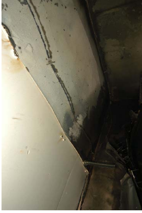
Figure 569 - View of the fire damaged wiring above the fire's area of origin.
