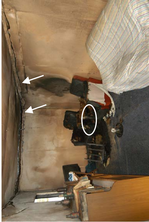
Figure 74 - Post-fire photograph of the view above showing the area of origin. The arrows indicate arcing damage locations.
