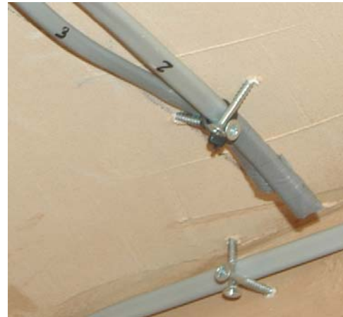
Figure 44 – The method of crossing two screws into an 'X' shape to support the cables during the fire and its suppression by fire crews.
