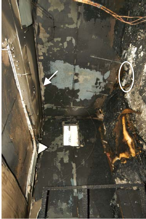
Figure 5 - Post-fire photograph. The white oval indicates the fire's area of origin. The white arrow indicates location of exhibit 001.
