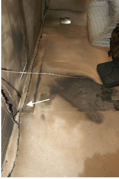
Figure 75 - Post-fire photograph detailing the location of exhibit 009 indicated by the white arrow.
