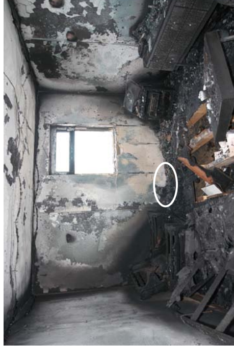
Figure 537 - Post fire photograph detailing the fire's area of origin. The floor has failed just in front of the remains of the Christmas tree.
