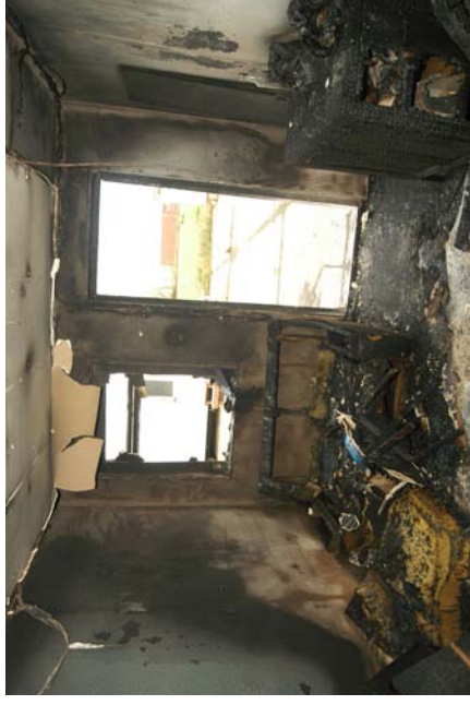
Figure 460 - Post-fire photograph of the front area of the compartment adjacent to the entrance door.
