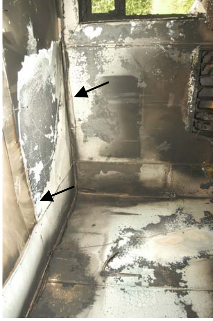
Figure 688 - Post-fire view of the fire's area of origin. The black arrows indicate the arcing damage to circuit 1 (R) and circuit 4 (L).
