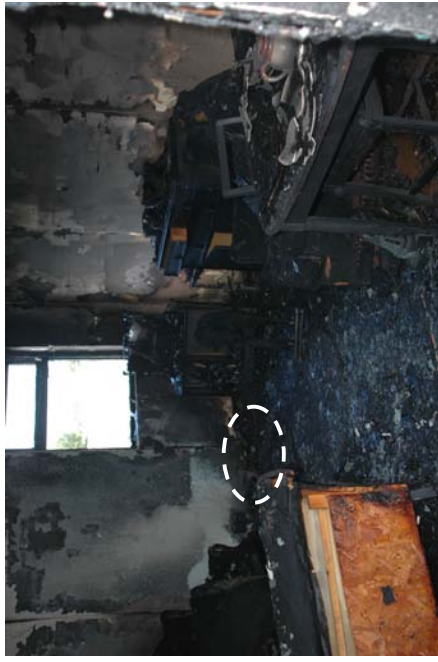
Figure 869 - Post-fire photograph with the area of origin detailed with a white dashed line oval.
