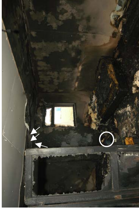
Figure 365 - Post-fire photograph with a white circle indicating the area of origin. The left arrow is the arcing damage to circuit 1. The middle and right arrows are the arcing damage to circuit 4.
