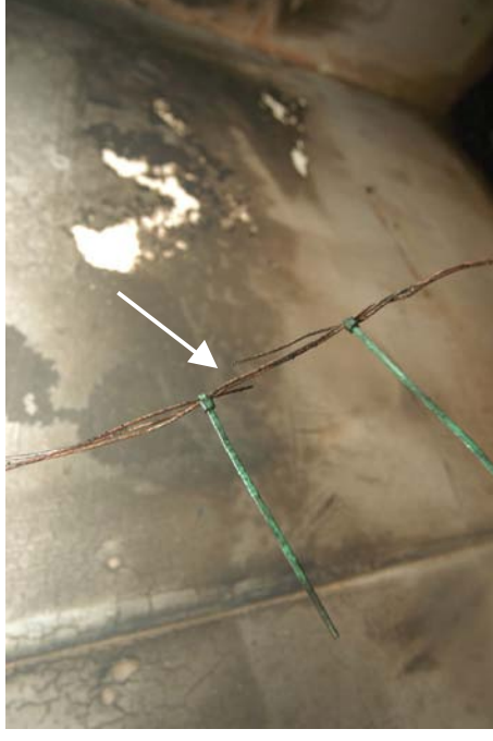
Figure 709 - A close-up photograph of the cable ties used during the electrical examination to identify the arcing damage to circuit 4.
