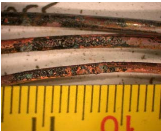
Figure 35 – Arcing through char affecting two conductors over a length of 14mm. The scale in the image is in mm.
