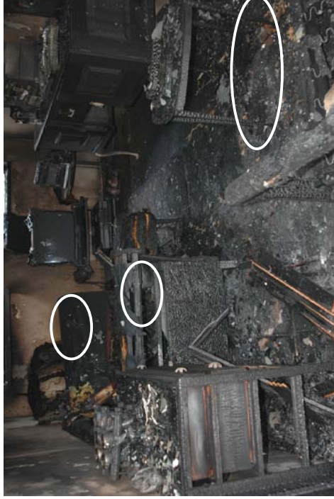
Figure 771 - Post-fire photograph taken from the entrance door.
