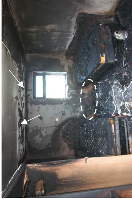
Figure 627 - Post-fire photograph, a 'U' shaped burn pattern was visible on the rear wall. Arcing damage was located above the area of origin on circuits 1 and 4 and is indicated by the white arrows.
