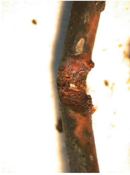
Figure 166 - Close-up view of the top conductor detailed in figure 164
