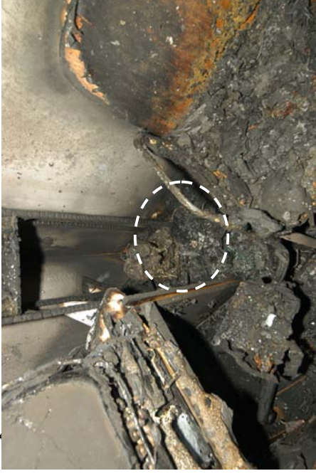
Figure 567 - Close-up view of the fire's area of origin – the rear left corner of the compartment.
