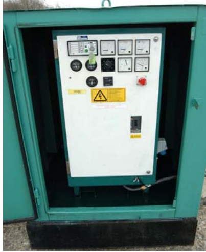
Figure 40 – The generator controls.
