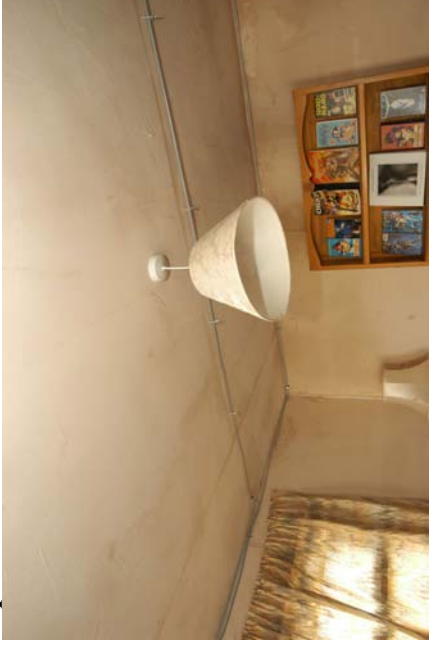
Figure 664 - View of the ceiling above the rear left corner of the compartment. Circuit 1 is the ring routed along the top of the walls and circuit 4 crosses the ceiling.
