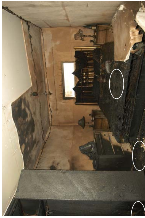
Figure 217 - Post-fire photograph the white ovals details detail the area of origin.
