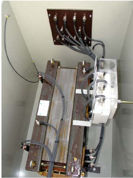
Figure 49 – The interior of the transformer.
