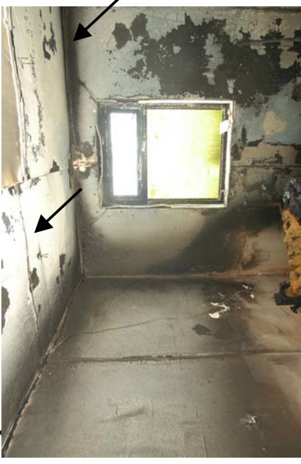
Figure 707 - Post-fire photograph of the ceiling area above the fire's area of origin. The left arrow indicates the arcing damage to circuit 4. The right arrow indicates the arcing damage location to circuit 1.
