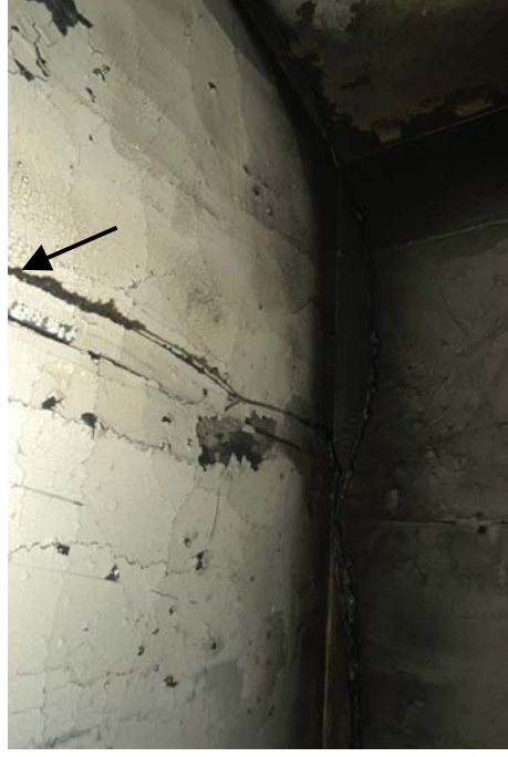
Figure 538 - Post-fire photograph of the rear left corner of the ceiling above the fire's area of origin. The arrow indicates circuit 4 that was routed across the ceiling.
