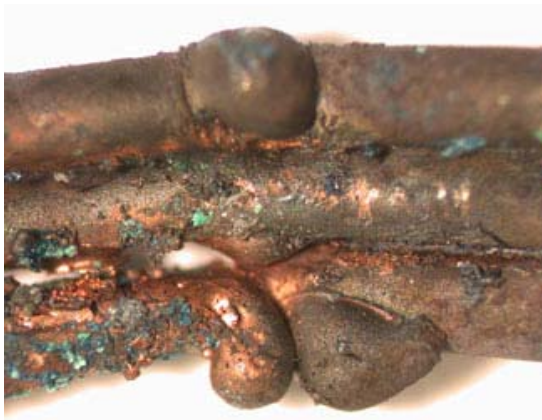
Figure 33 – Gross beading affecting all three conductors of this cable. The conductors are also welded together.
