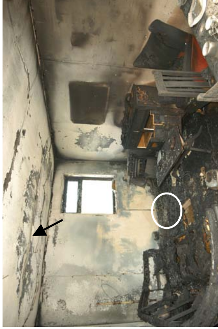
Figure 648 - Post-fire photograph detailing the fire's area of origin. The black arrow was the location of the arcing damage to circuit 4 above the fire's area of origin.
