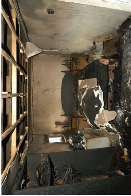
Figure 271 - Post-fire over-view image of experiment 13. Most of the ceiling plaster board fell down shortly after the fire was extinguished.
