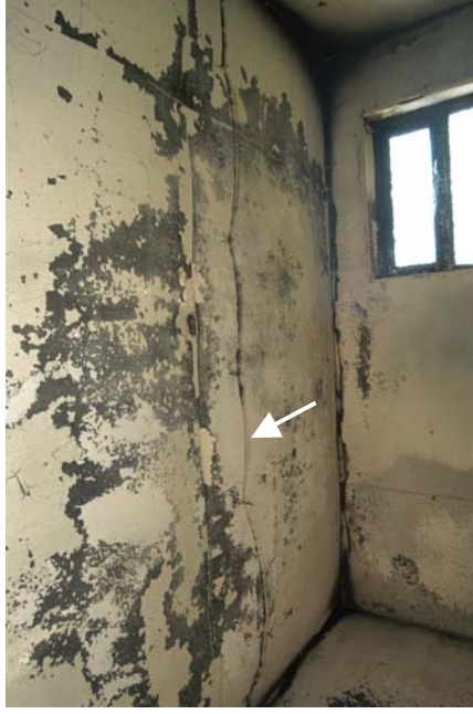
Figure 649 - Post-fire photograph of the ceiling area above the fire's area of origin. The white arrow details the arcing damage location of circuit 4 - exhibit 097.
