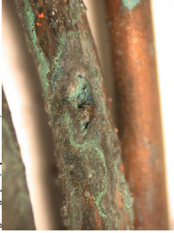
Figure 694 - A close-up of the arcing damage to this conductor, the middle conductor detailed in figure 693.
