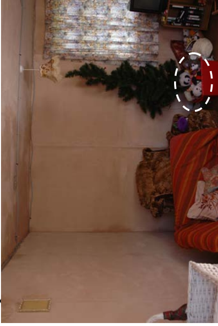
Figure 868 - The ceiling and wiring above the area of origin.
