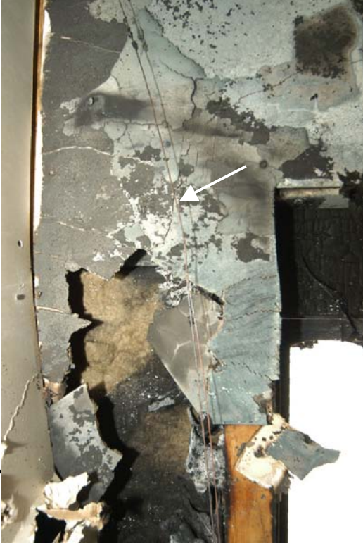
Figure 198 - Arcing damage to exhibit 029 on circuit 1.
