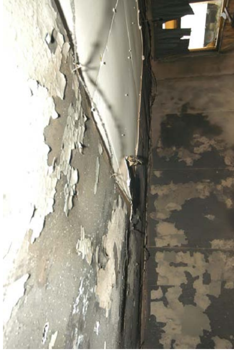
Figure 366 - Post-fire photograph the ceiling area of the front of the compartment. This details circuits 1 (wall edge), 2 and 3 (routed across the ceiling).
