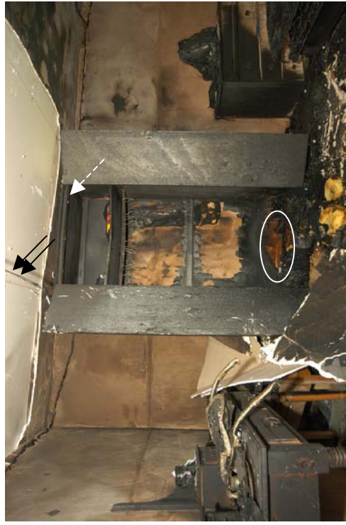
Figure 218 - Post-fire photograph of the wardrobe area in the compartment. The arrows indicate areas of arcing.
