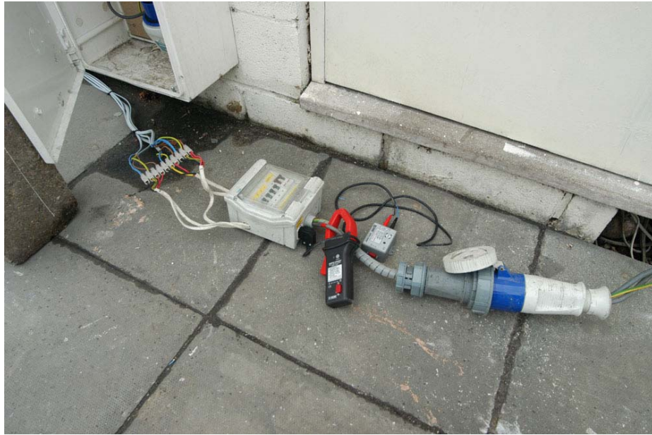
Figure 56 – The voltage and current loggers connected to the research circuits.
