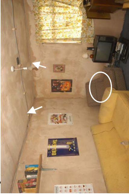
Figure 901 - Pre-fire photograph detailing the wiring installed on the ceiling using wooden blocks. The arrows indicate the arcing locations to circuit 4 (L) and circuit 1 (R).
