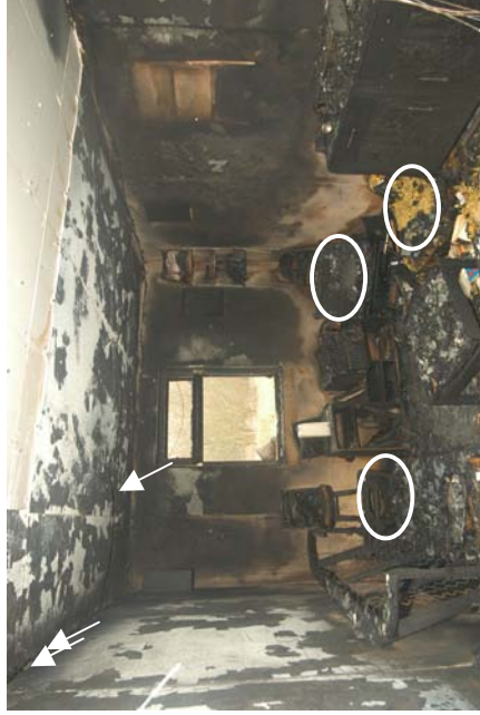
Figure 404 - Post-fire photograph with white ovals indicating the three points of origin. The right arrow locates the arcing damage to circuit 4. The middle arrow indicates the second area of arcing to circuit 4, the left arrow indicates the arcing damage to circuit 1.
