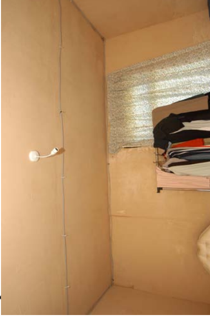
Figure 626 - Pre-fire photograph detailing the electrical circuits fixed to the ceiling above the area of origin.
