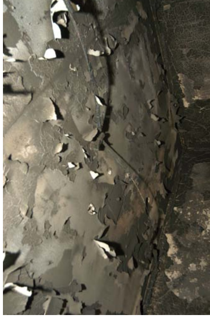
Figure 983 - Post-fire view of the ceiling above the fire's area of origin and the armchair located in the left rear corner of the compartment.
