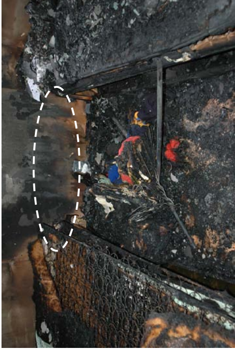
Figure 835 - Close-up view of the fire's area of origin. Arcing damage to circuits 1 and 4 was located above this area on the ceiling.
