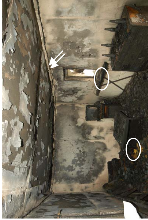
Figure 245 - Post-fire photograph with the white ovals indicating the fire's areas of origin and the arrows indicating points of arcing to circuits 1 and 4.
