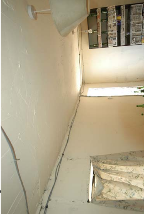
Figure 244 - Pre-fire photograph of the wiring installed on the ceiling for the experiment.
