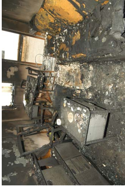
Figure 336 - Post-fire photograph of the view shown above in figure 334.
