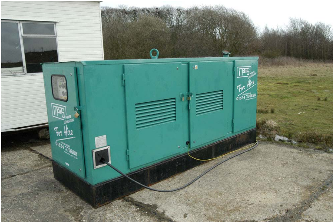
Figure 39 – The 60 kVA three-phase generator on site.
