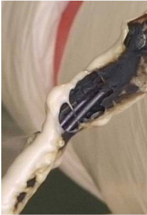
Figure 15 – Current overloaded PVC insulated cable [45].
