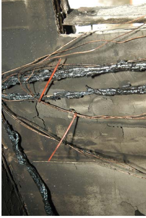
Figure 6 - Post-fire photograph indicating the arcing damage to circuit 3 above the doorway.
