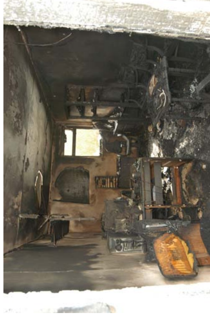
Figure 482 - Post-fire photograph of the compartment.
