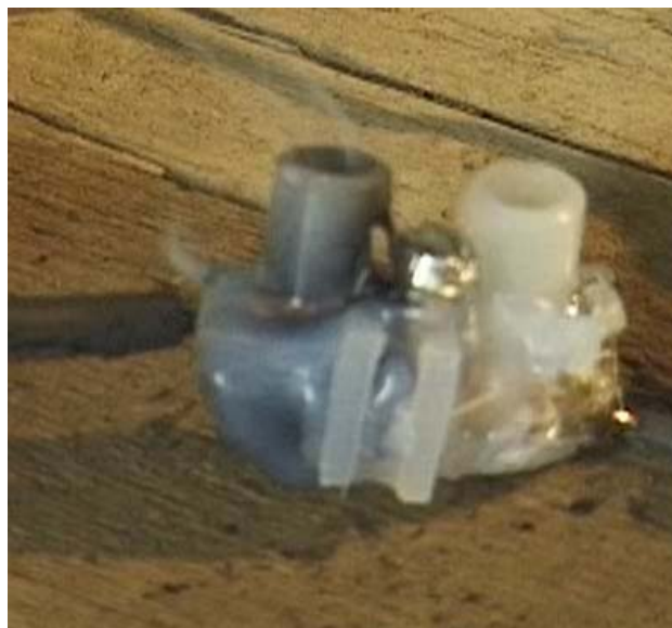
Figure 17 – Resistance heating of a terminal connection [45].
