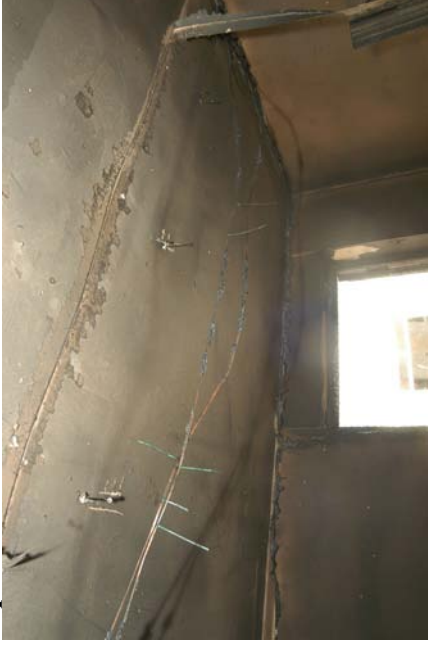
Figure 742 - Post-fire photograph of the ceiling detailing circuits 2 and 3.
