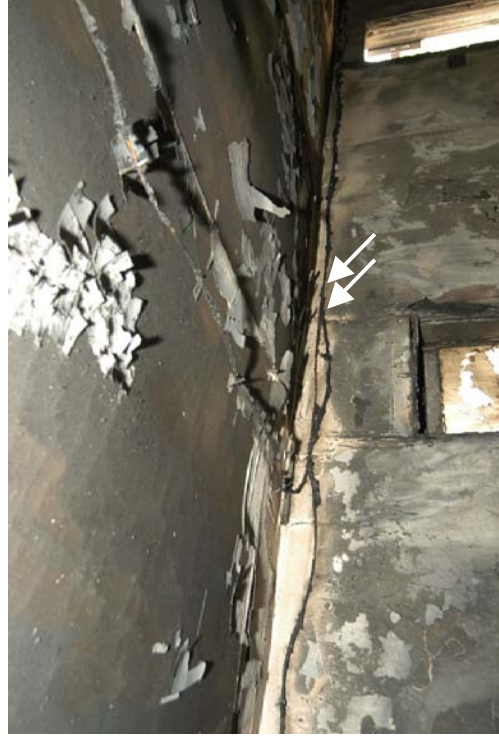
Figure 246 - Post-fire photograph of the ceiling with arrows indicating points of arcing at circuits 1 and 4.
