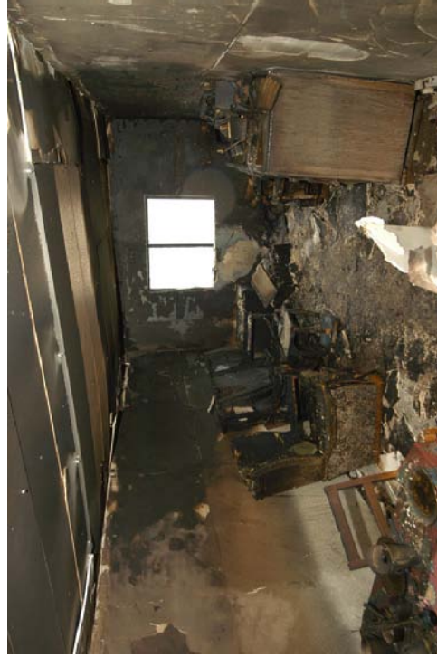
Figure 136 - Post fire photograph of experiment 7, burn patterns show protected areas at low level.
