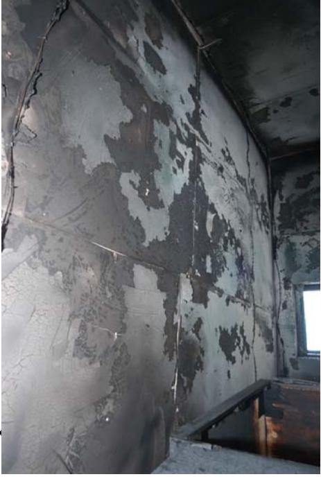
Figure 506 - Post-fire photograph of the ceiling above the fire's area of origin.
