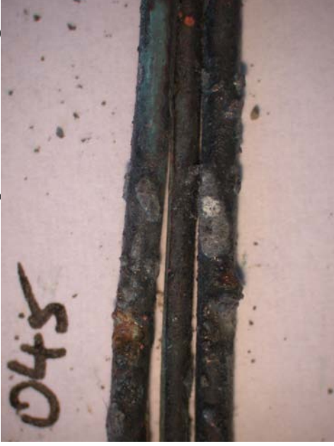
Figure 299 - Microscope image of exhibit 045, two of the conductors have notch damage.
