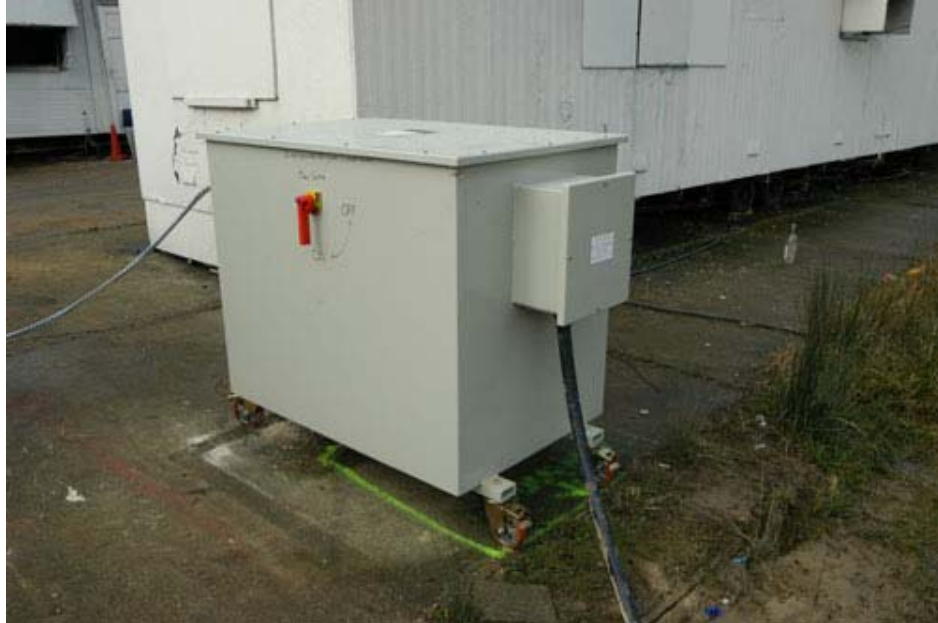
Figure 48– The 75kVA transformer installed on-site.
