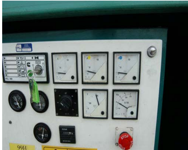
Figure 41 – The electrical output of the generator is displayed with voltage, current and frequency meters that are built into the control panel.
