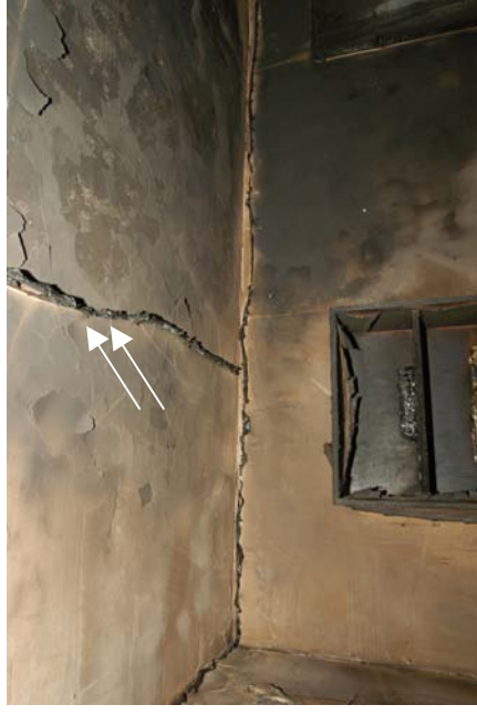
Figure 314 - Post-fire view of the fire damaged wiring above the dominant area of origin, the shelf unit. The arrows indicate the arcing damage to circuits 2 and 3.
