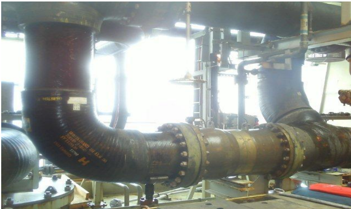
Fig. 1.4: Application of Fiber Reinforced Plastic (FRP) on an Offshore Facilities at Gulf of Guinea.
