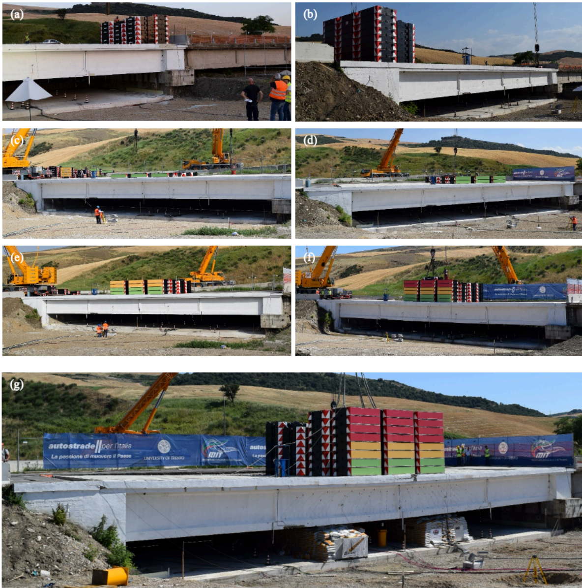
Figure 4.10 Pictures of the Alveo Vecchio viaduct during the loading phases (a) PP – 4800 kN; (b) PA – 4800 kN; (c) P1 – 1200 kN, (d) P2 – 2400 kN, (e) P3 – 4800 kN, (f) P4 – 7200 kN, and (g) P5 – 9600 kN
