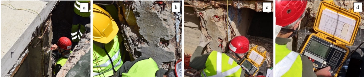
Figure 6.11 a) Inspector cleaning the rust from the steel wires with a metallic brush; (b) the cleaned steel cables ‘anchors; (c) Inspectors performing RIMT; (d) real-time outcome.
