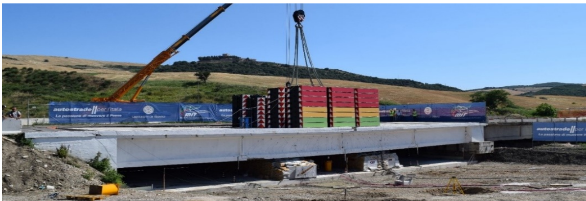
Figure 5.9 The Alveo Vecchio viaduct during the loading phase 5, loaded with 93 weights—9300 kN.
