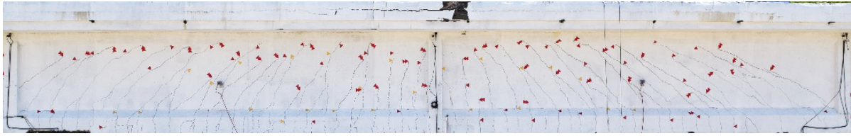
Figure 4.15 Visible cracks on the middle portion of girder T4 opened during the loading phases P3 (amber triangles), P4 (red single triangles), and P5 (red double triangles)
