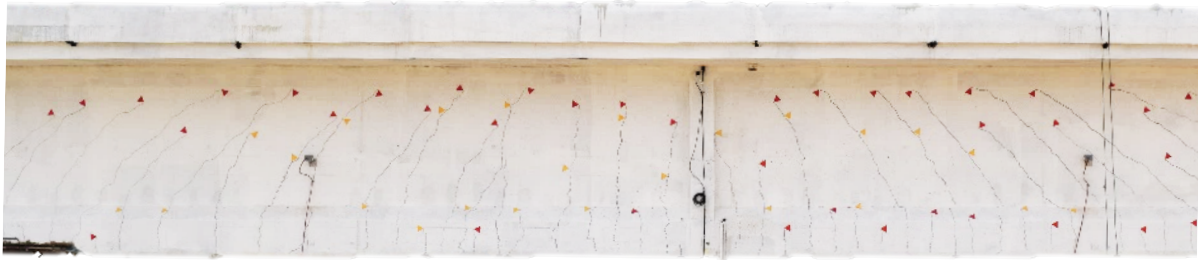
Figure 5.13 Visible cracks on girder T1 opened during the loading phase P4 7200 kN.
