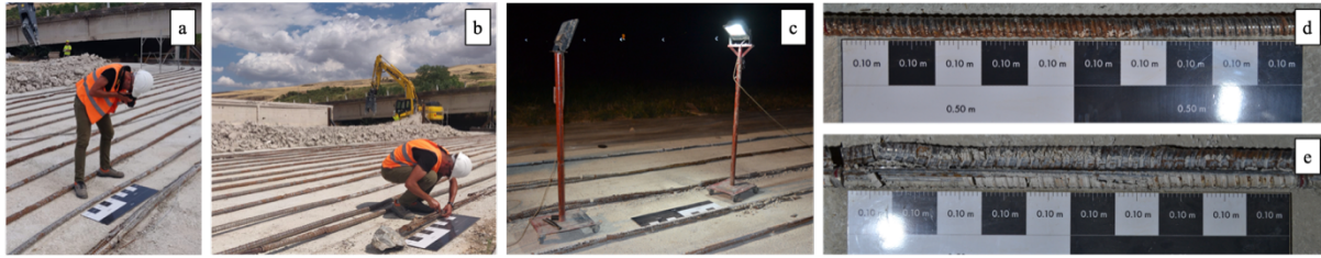
Figure 3.3 (a and b) Mapping activity of the actual condition state of a prestressing cable; (c) procedure adopted during the night; (d) 1 m long ruler positioned for mapping the condition state of the metal duct; (e) 1 m long ruler positioned for mapping the condition state of the injected grout and the steel cable.
