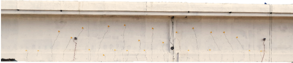
Figure 5.12 Visible cracks on girder T1 opened during the loading phase P3 4800 kN.
