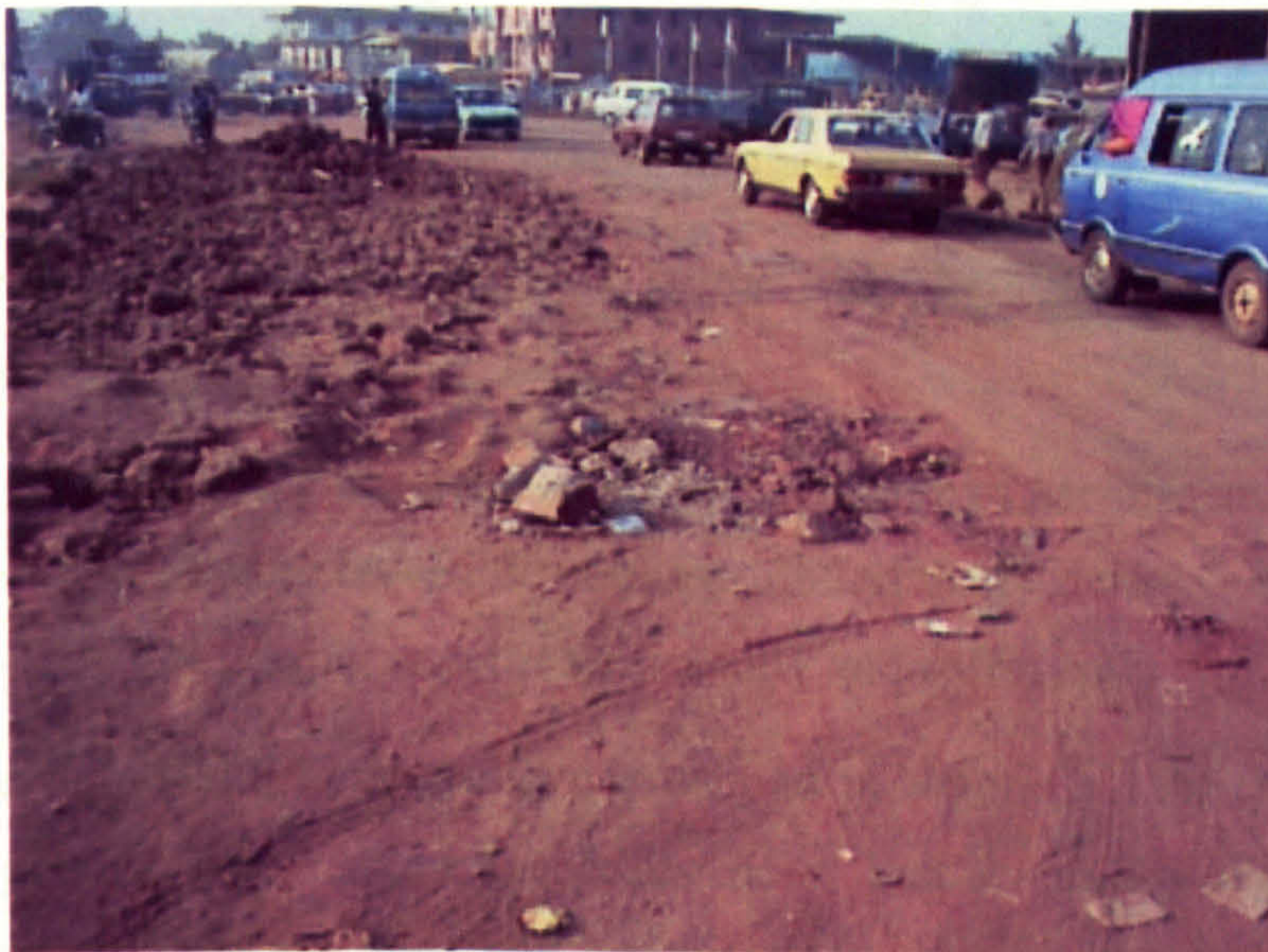
Figure 3.3 Typical Road Distress.
