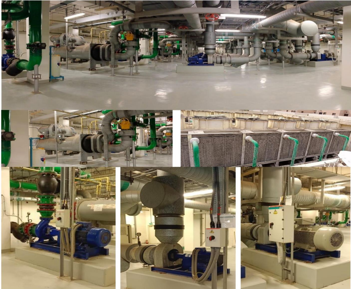
Figure 18: Panoramic view of chilled water system
