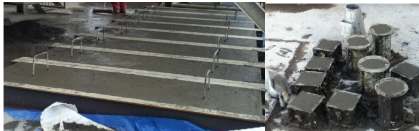
Figure 9.6: Typical Beams for Series "2" together with own Control Samples after Concrete Casting.
