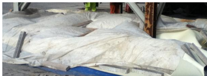
Figure 7.7: The Curing Process of Typical Beams in Series "1" after Removing the Shutters.
