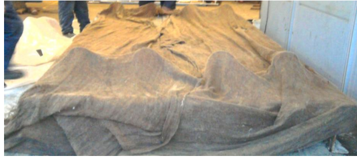
Figure 5.7: The Curing Process of the Beams in Series "A" after Removing the Shutters.
