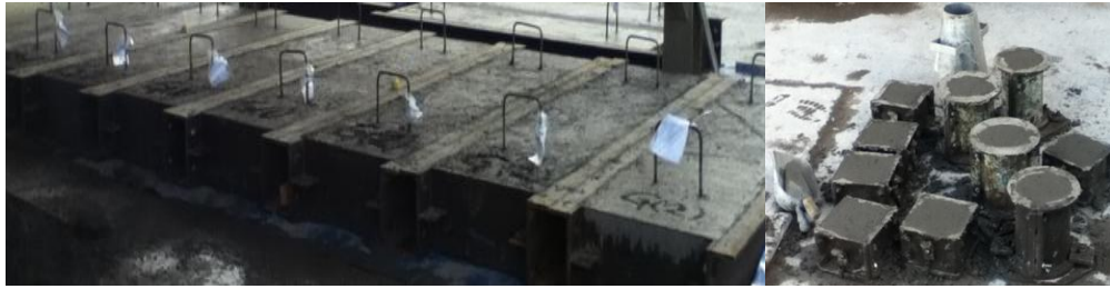
Figure 7.6: Typical Beams for Series "1" together with own Control Samples after Concrete Casting.
