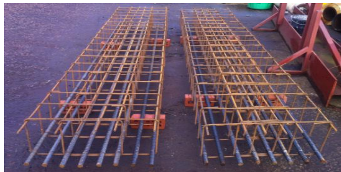
Figure 5.4: Steel Cages of the Beams in Test-Series "A"; From Left: Beams ECC2 and ECC3.
