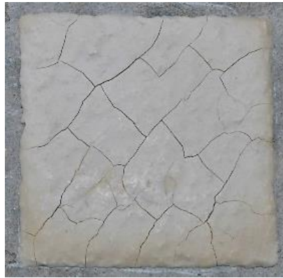
Figure 5.8 – Cracked patch printed onto dry concrete substrate.
