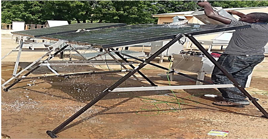
Figure 4-19 Spraying of PV module with cold water.
