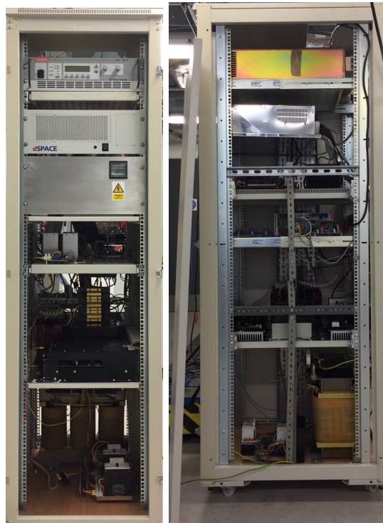
Figure 3.1: Pictures of the 10 kVA inverter with customizable control strategy (front and side view).
