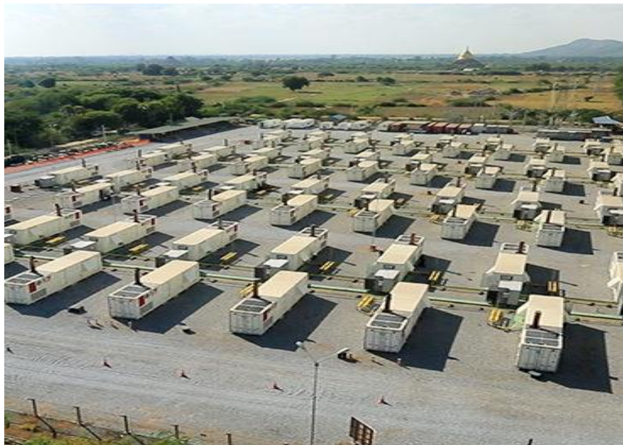
Figure 3: Fossil fuel-based power generators (APR Energy, 2018).
