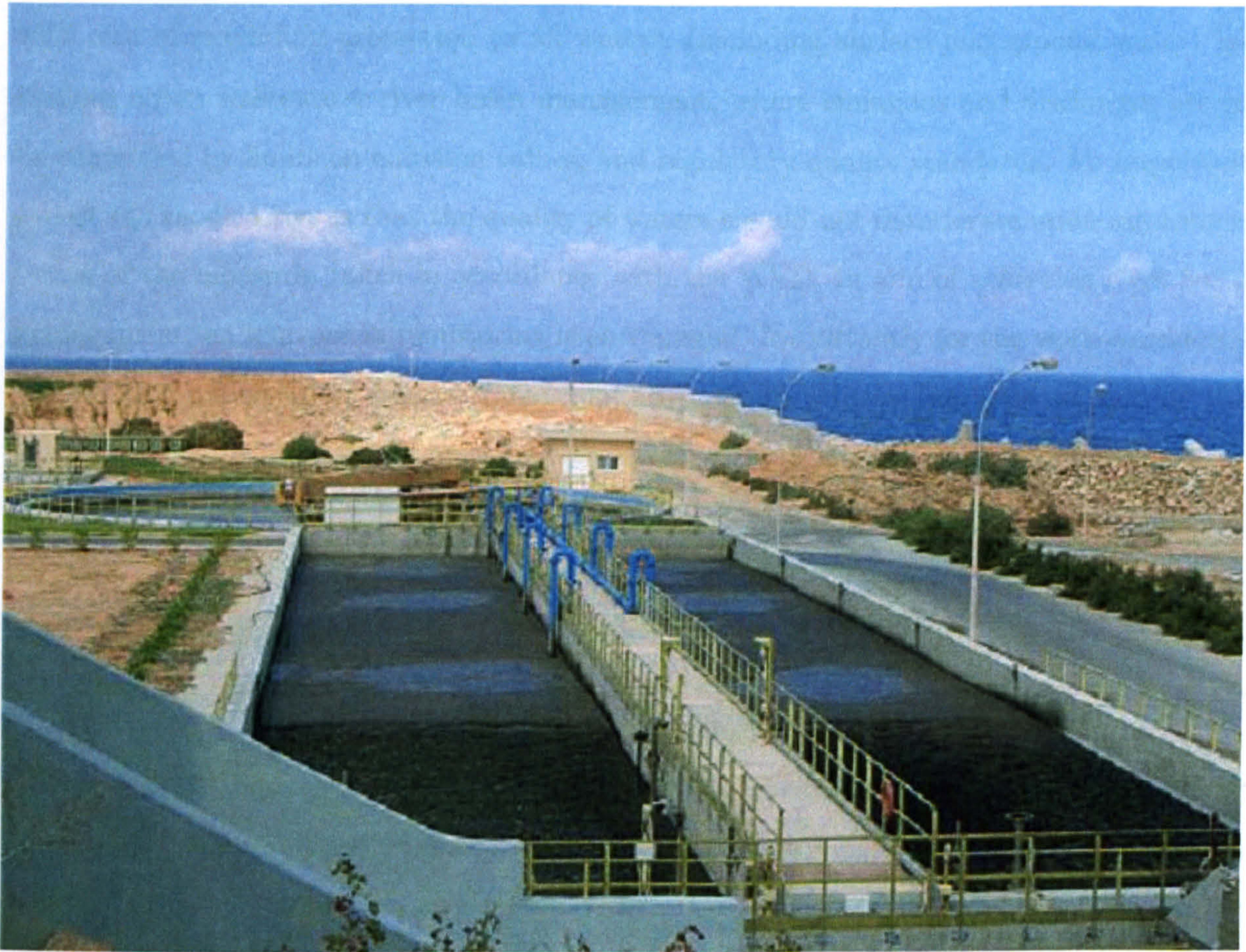
Figure 1-3: Aerated Activated Sludge Detention Tanks in a Wastewater Treatment Plant: Foreground: The Aerated Activated Sludge Tanks, Background The Secondary Clarifier.
