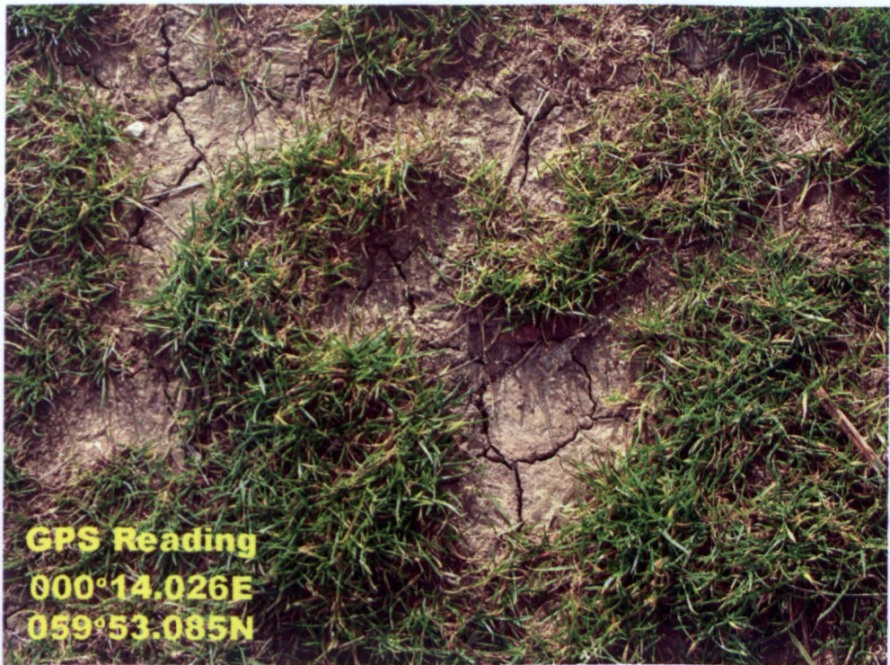
Figure 3.9 Pattern of desiccation cracks observed on the crest of the new embankment (2006).
