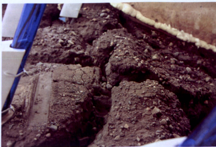
Figure 8.17 5 cm deep cracks on the crest edge after first day of flooding.
