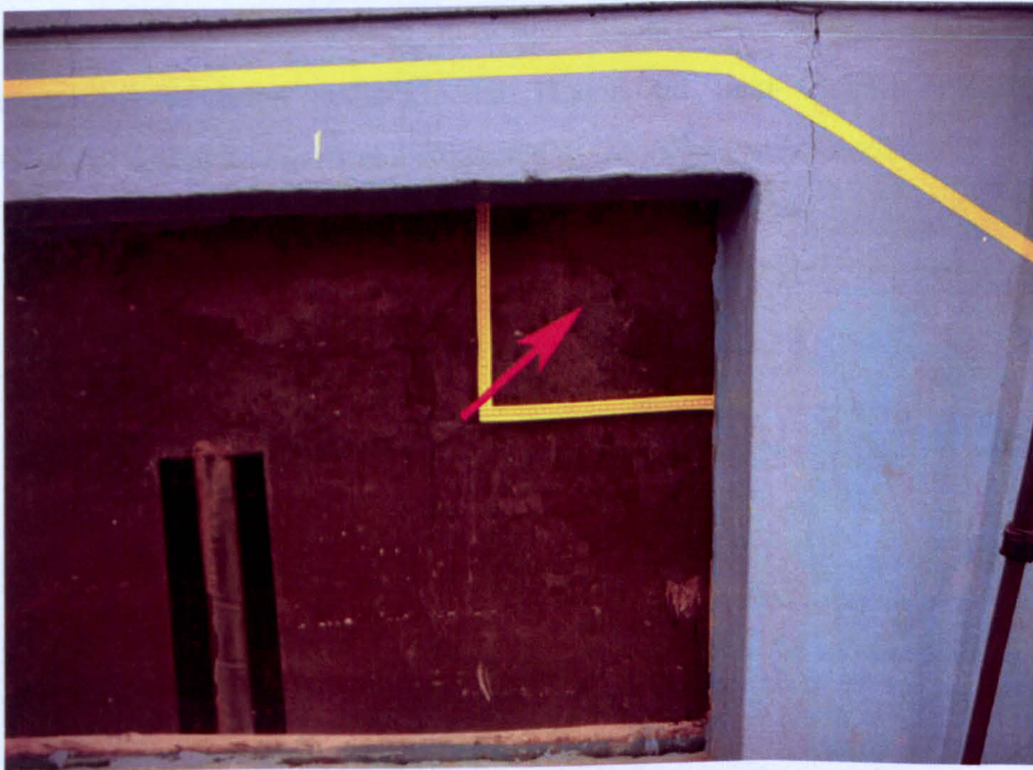
Figure 7.38 Crack parallel to the slope.
