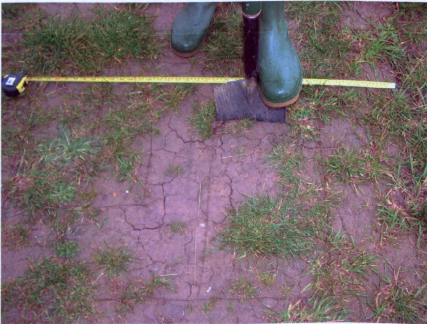
Figure 3.13 Photograph of surface desiccation fissuring on crest of new embankment prior to hand excavation (2006).
