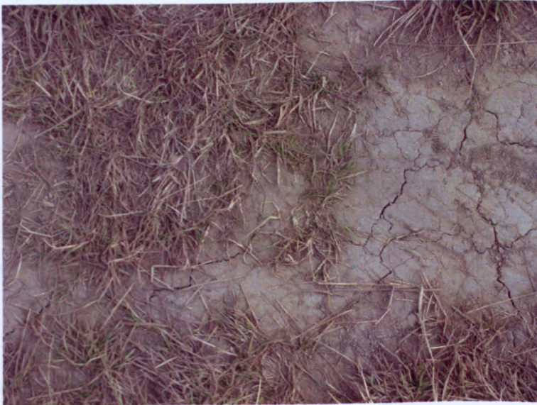
Figure 3.37 Cracks visible on the crest surface, Lancaster.
