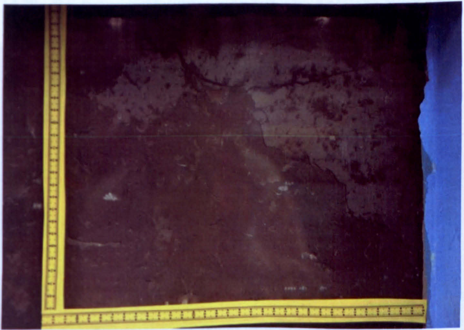
Figure 14.27 Crack parallel to the slope.
