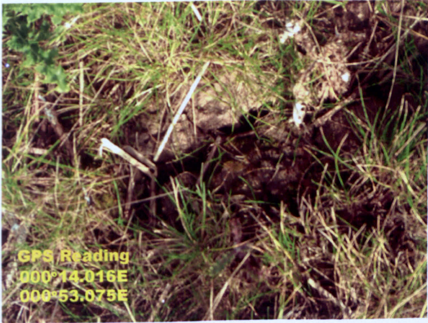
Figure 14.4 Crack on the slope.
