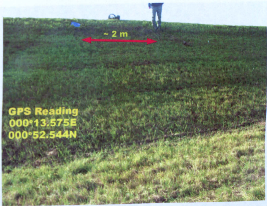
Figure 14.6 Crack on the slope with the length.
