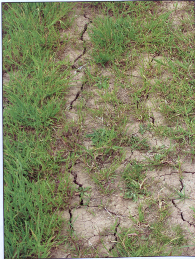
Figure 3.11 Pattern of desiccation and differential fissures observed along crest of new embankment (2006).
