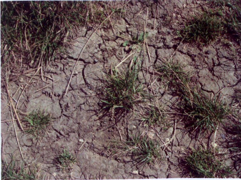
Figure 3.29 Superficial cracking observed at Windsor embankment.
