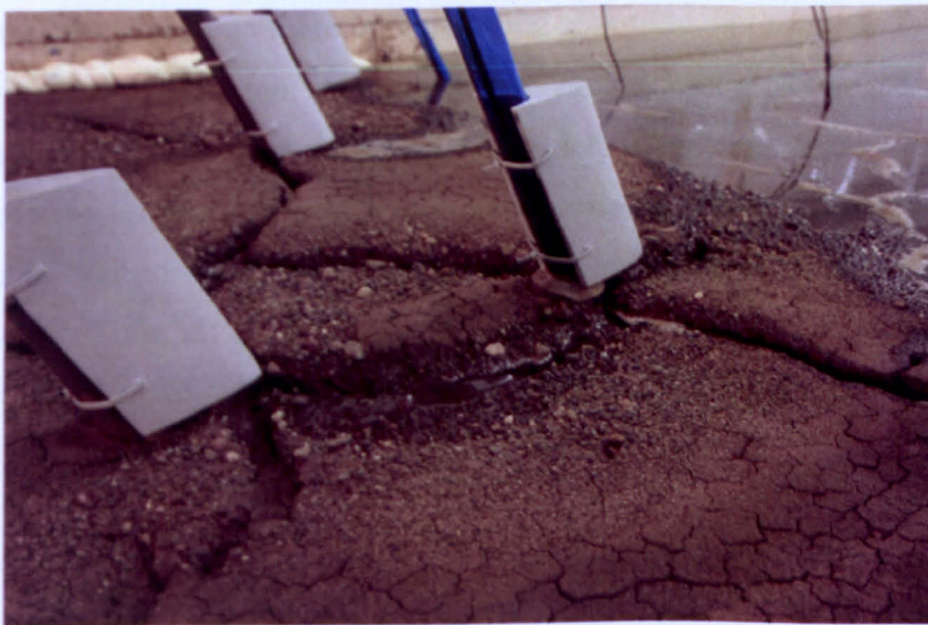
Figure 8.12 Water penetrating cracks on the crest.
