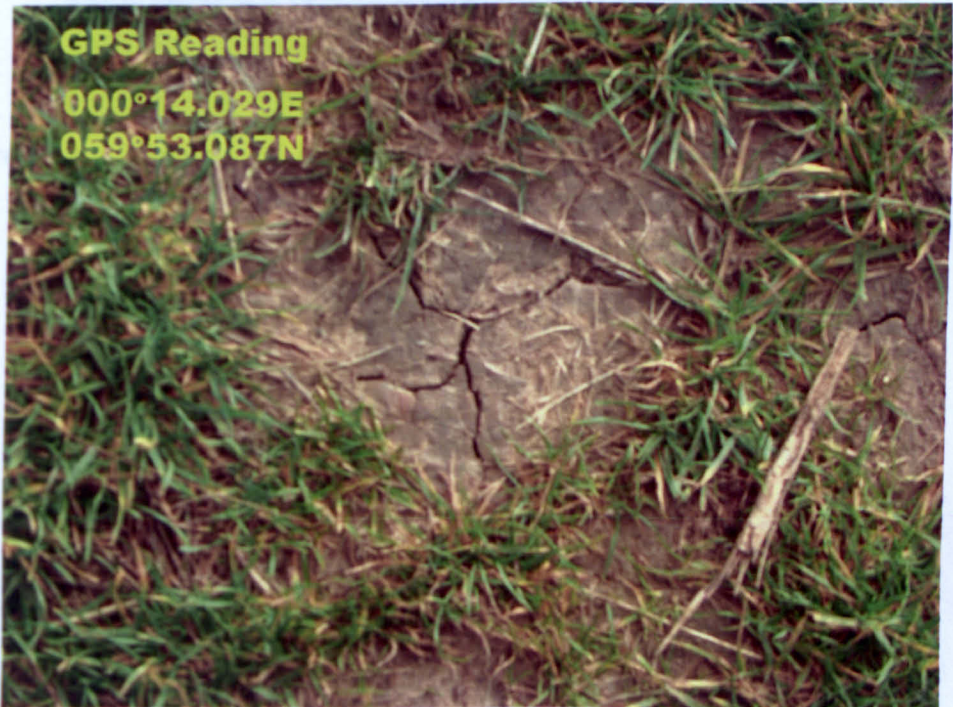
Figure 14.1 Cracks on the crest.
