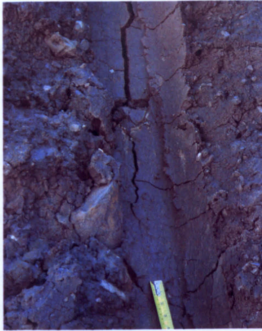
Figure 4.1 State of desiccation cracking indicated in the quarry.
