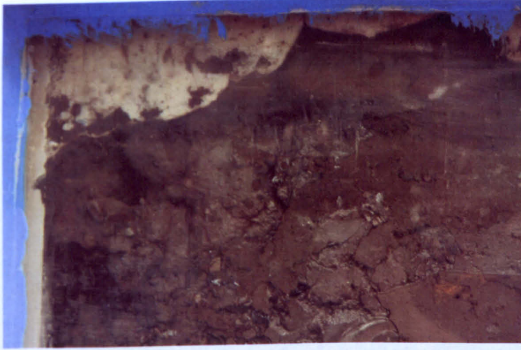
Figure 8.14 Eroded crack inside embankment close to the edge of the slope.
