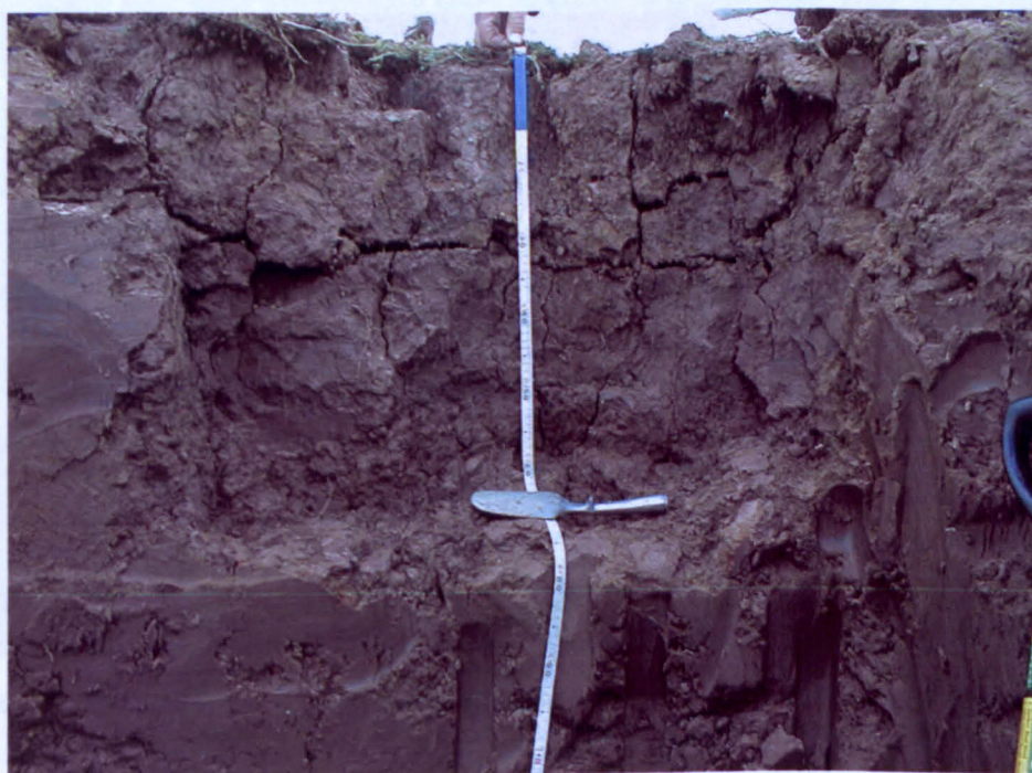
Figure 3.3 Desiccation fissures observed in trial trench at Thorngumbald flood embankment at an approximate depth of 600 mm below crest level (after Dyer et al. 2009).
