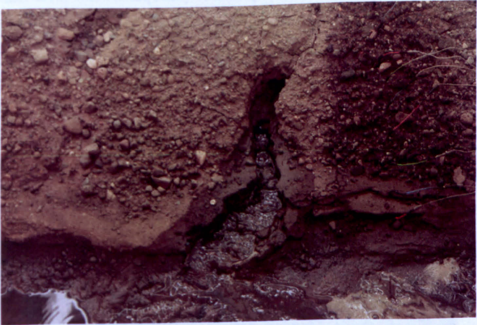
Figure 8.10 Local seepage from the bottom of the slope.
