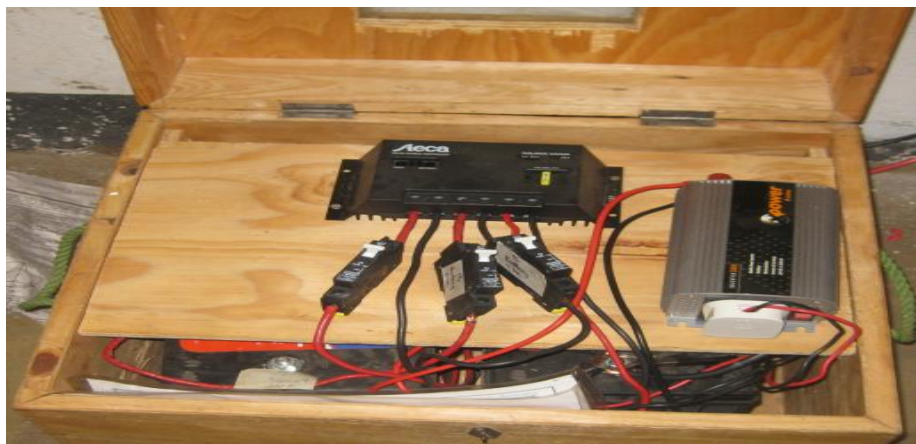
Figure 4. 12: Battery bank, Charge Controller and Inverter
