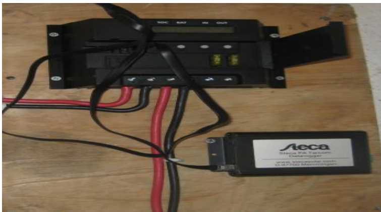
Figure 4. 11: Steca Tarom Data Logger and Charge Controller
