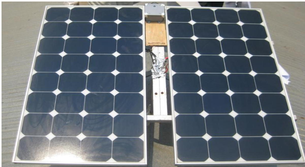
Figure 4. 10: Outdoor Solar PV Monitoring System Showing Mono-crystalline PV Modules and Radiation Sensor. Source: Authors own experimental set up and camera pictures
