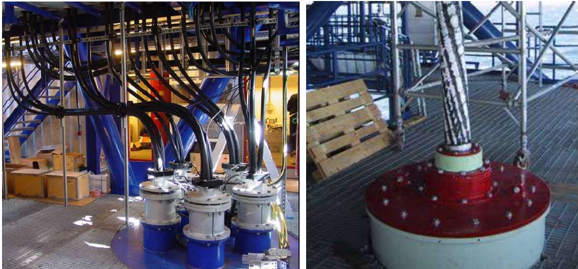
Figure 2.9. Armouring hang-off of the five inter-array 33kV cables and the 150kV export cable on the substation at Horns Rev.
