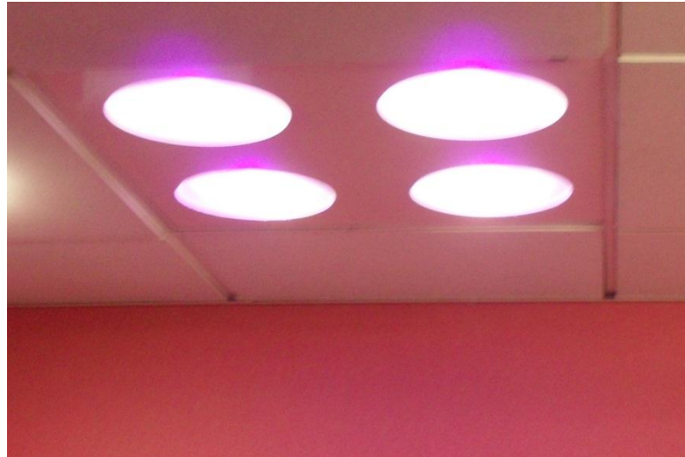
Fig. 9.40. Photograph of the new HINS-light EDS as a bank of four ceiling mounted light sources each with a diffuser and Fresnel lens.
